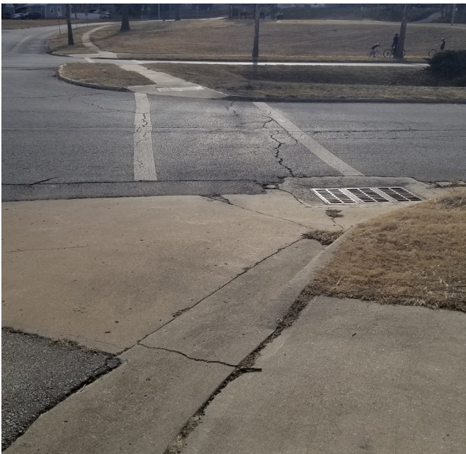
Mis-aligned ramp and crosswalk near McCoy Park
