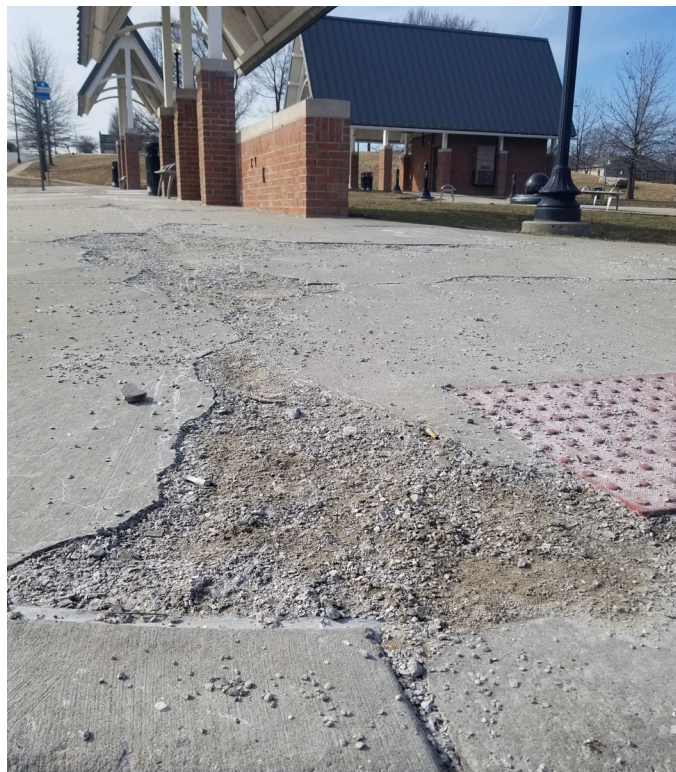
Poorly-maintained sidewalks can create a safety hazard for pedestrians and people using a wheelchair or other mobility device. (Independence Transit Center)
