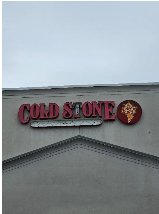
Figure 1: Degradation of External Finishes
