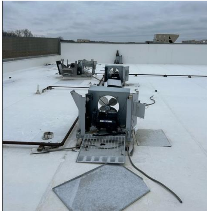
Figure 2: Destroyed HVAC Systems
