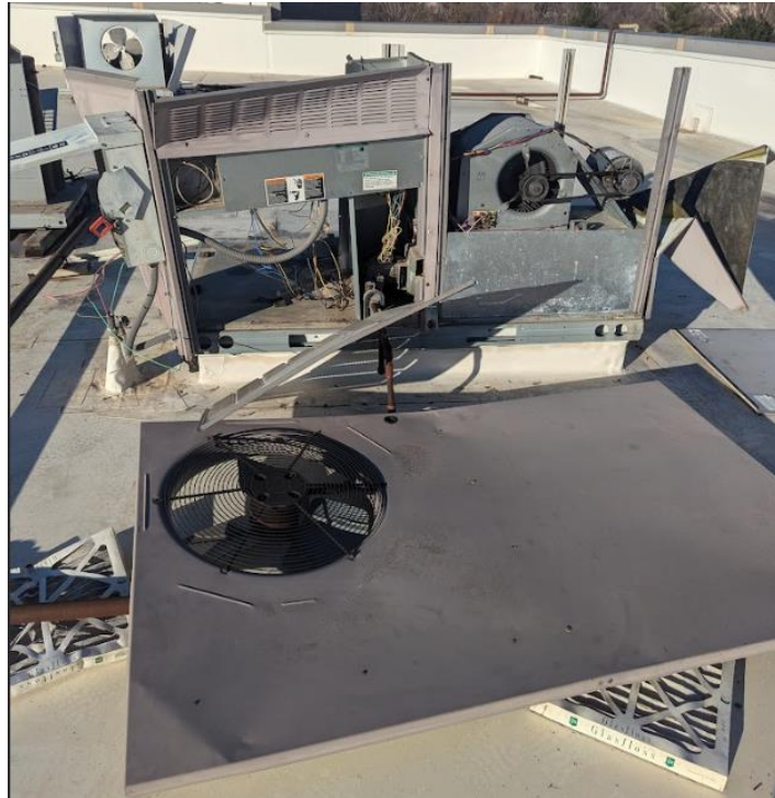
Figure 3: Destroyed HVAC Systems
