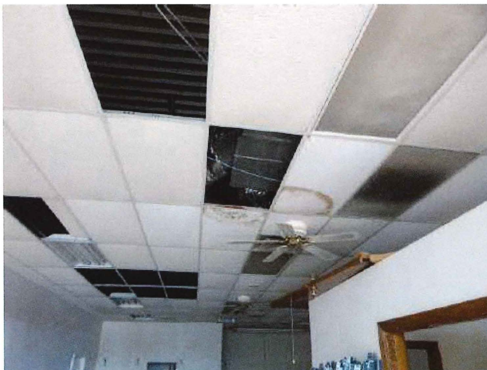
4378 S Noland Rd – roof leaks
