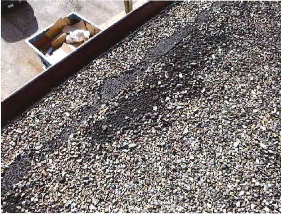
4452 S Noland Rd – worn gravel ballast
