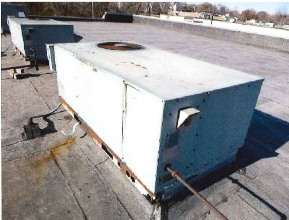
RTU at end of useful life
