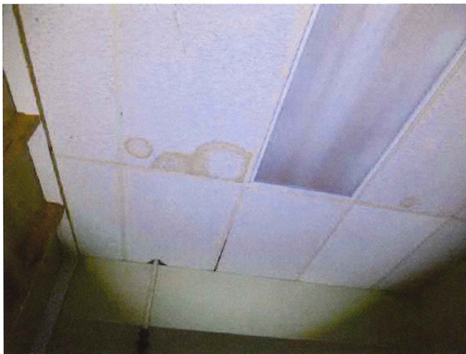
4374 S Noland Rd – roof leaks
