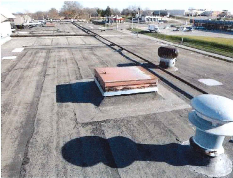
4466 S Noland Rd – lack of fall protection
