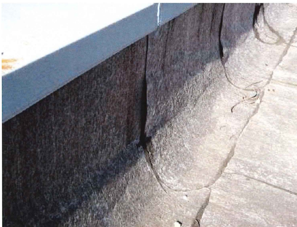
4510 S Noland Rd - Failing seams at west parapet
