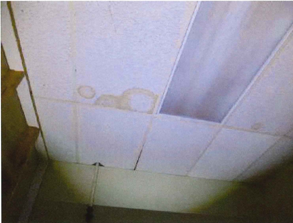
4374 S Noland Rd – roof leaks
