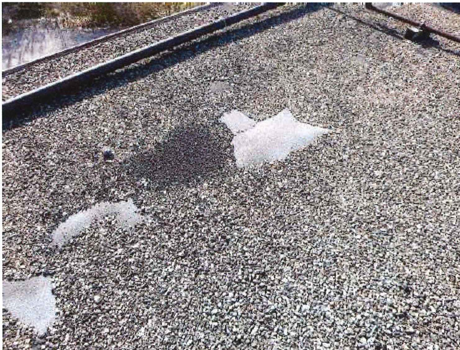
4452 S Noland Rd – bubble in roof
