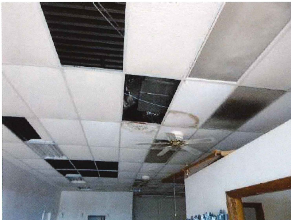
4378 S Noland Rd – roof leaks
