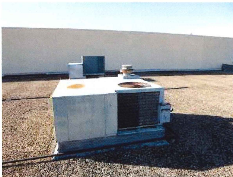
RTU installed in 1980s
