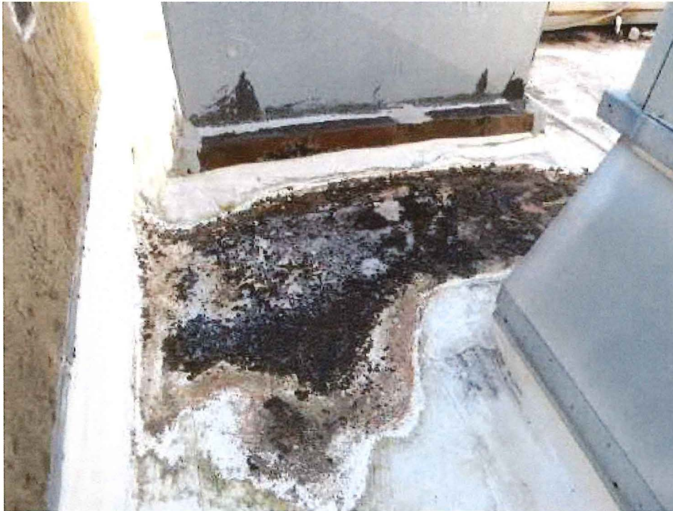
4400 S Noland Rd – ponding of water in area of leaking roof
