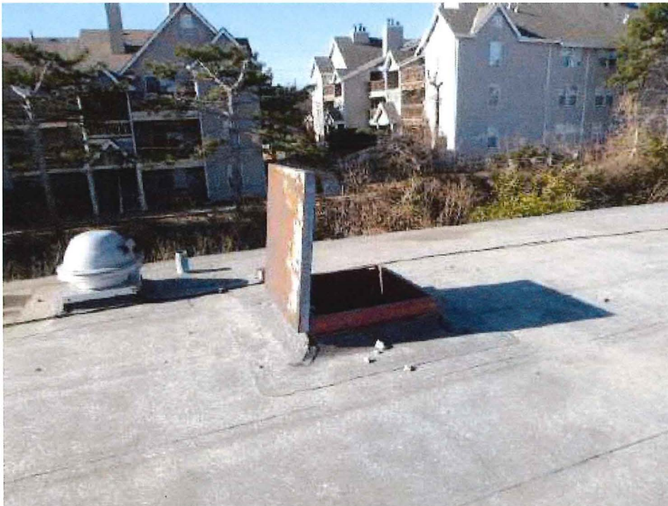
4420 S Noland Rd – lack of fall protection at roof hatch
