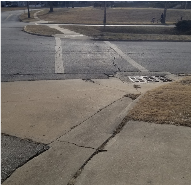
Mis-aligned ramp and crosswalk near McCoy Park
