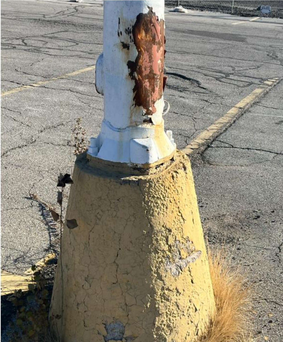
Deteriorated Light Pole
