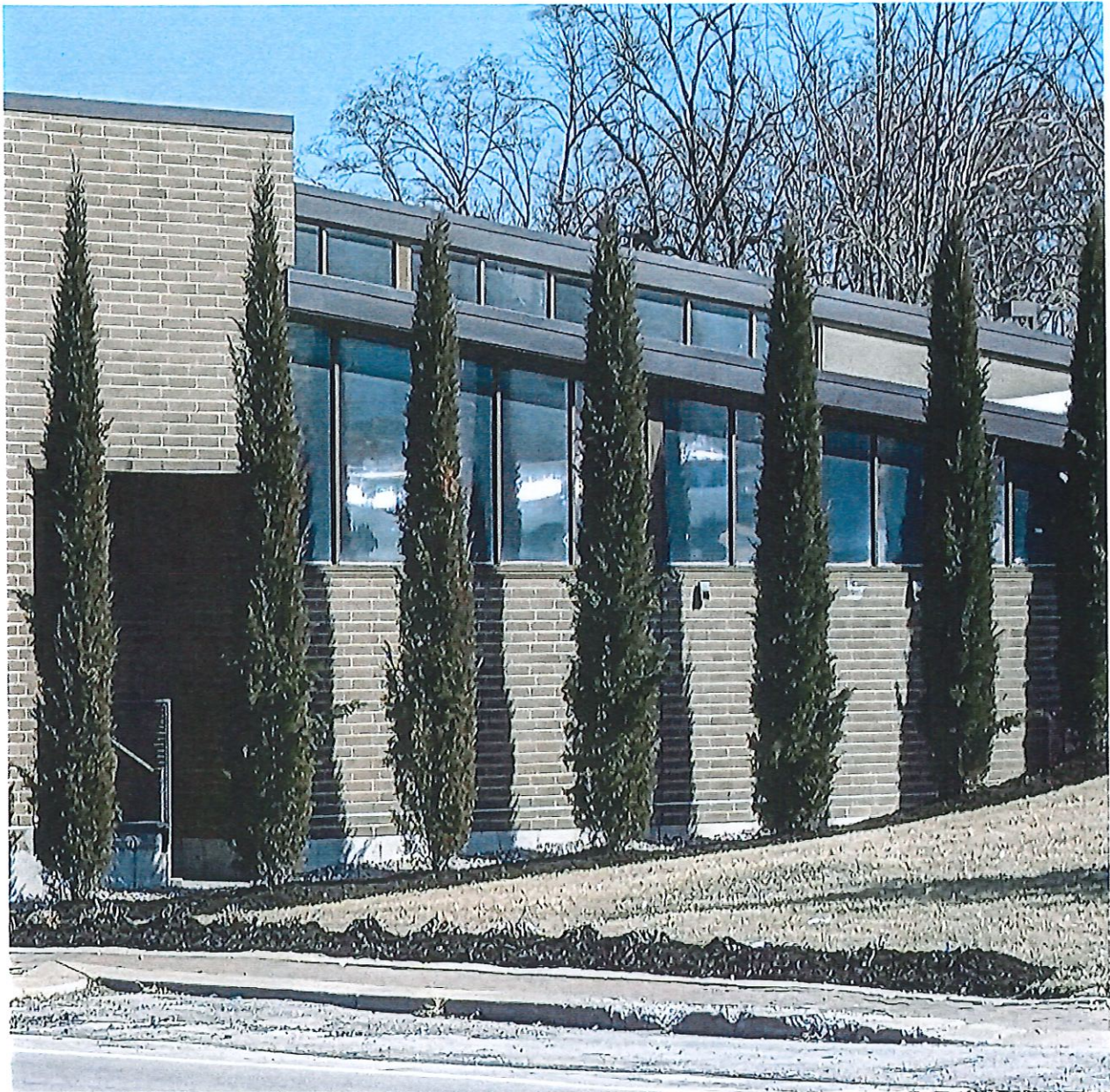
Parcel No. 27-120-07-36-00-0-00-000 Curbing deteriorating.
