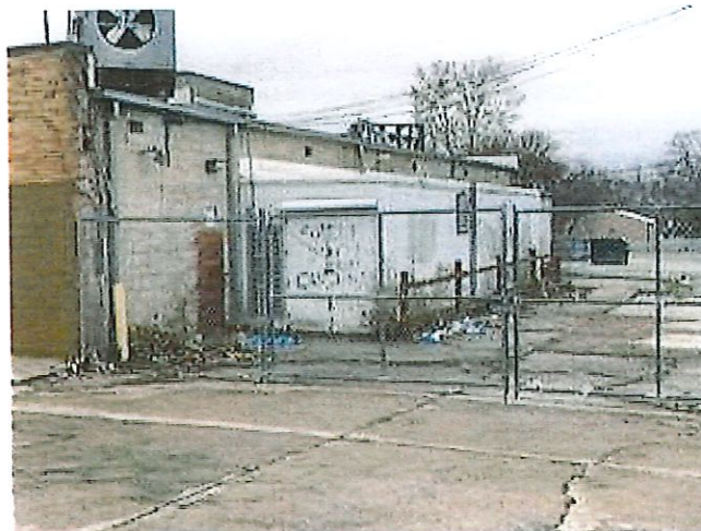
Parcel No. 15-940-04-10-00-0-000 Trash, broken driveway cement
