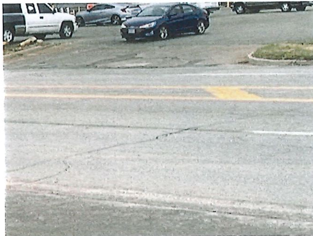
Parcel No. 15-940-04-09-00-0-00-000 Broken driveway pavement
