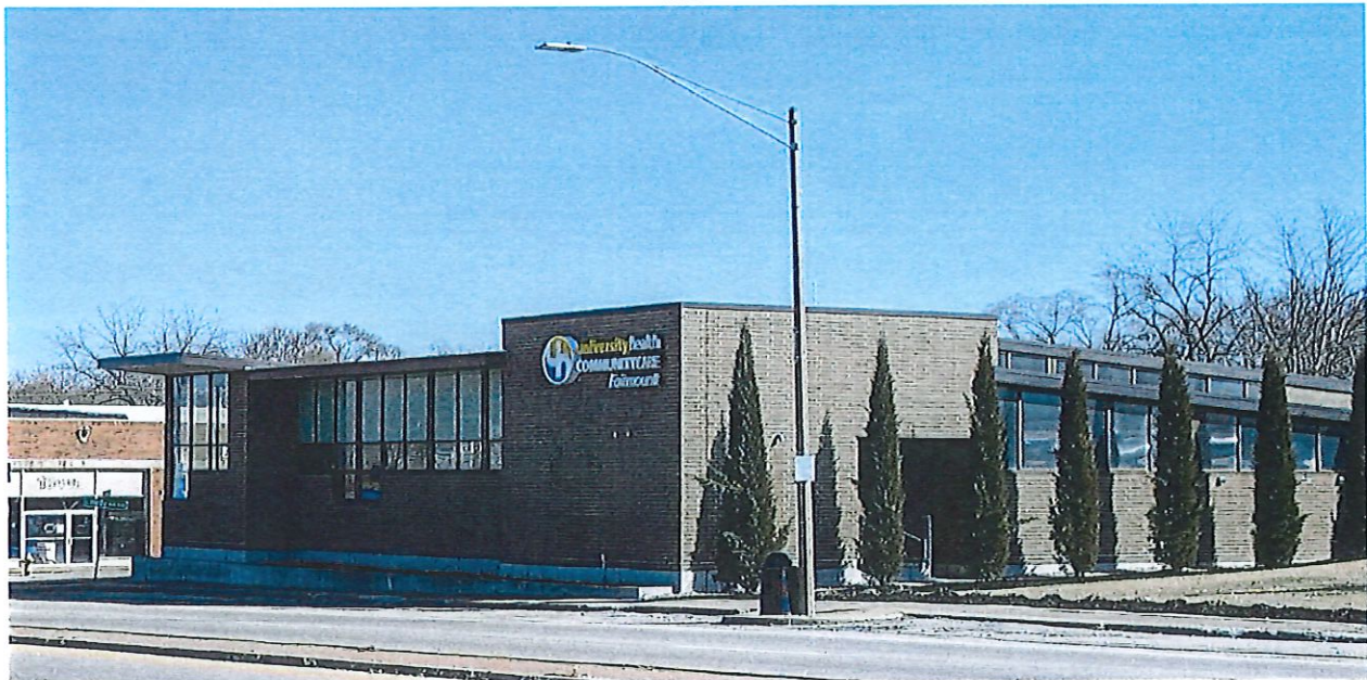
Parcel No. 27-120-07-36-00-0-00-000 Curbing deteriorating.
