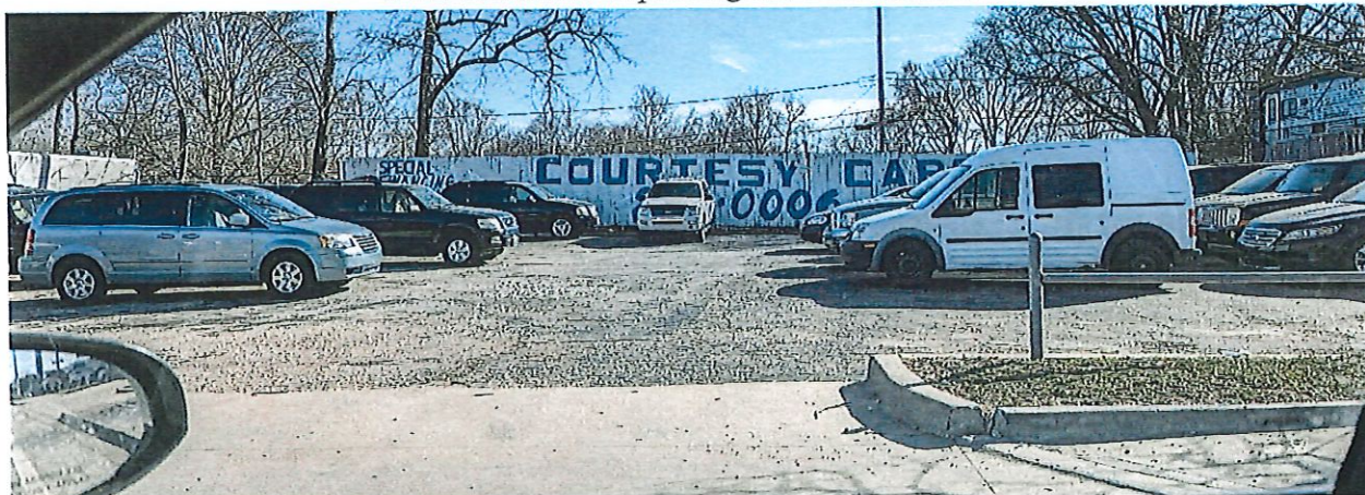
Parcel No. 27-120-02-05-00-0-00-000 Poor condition of parking lot.
