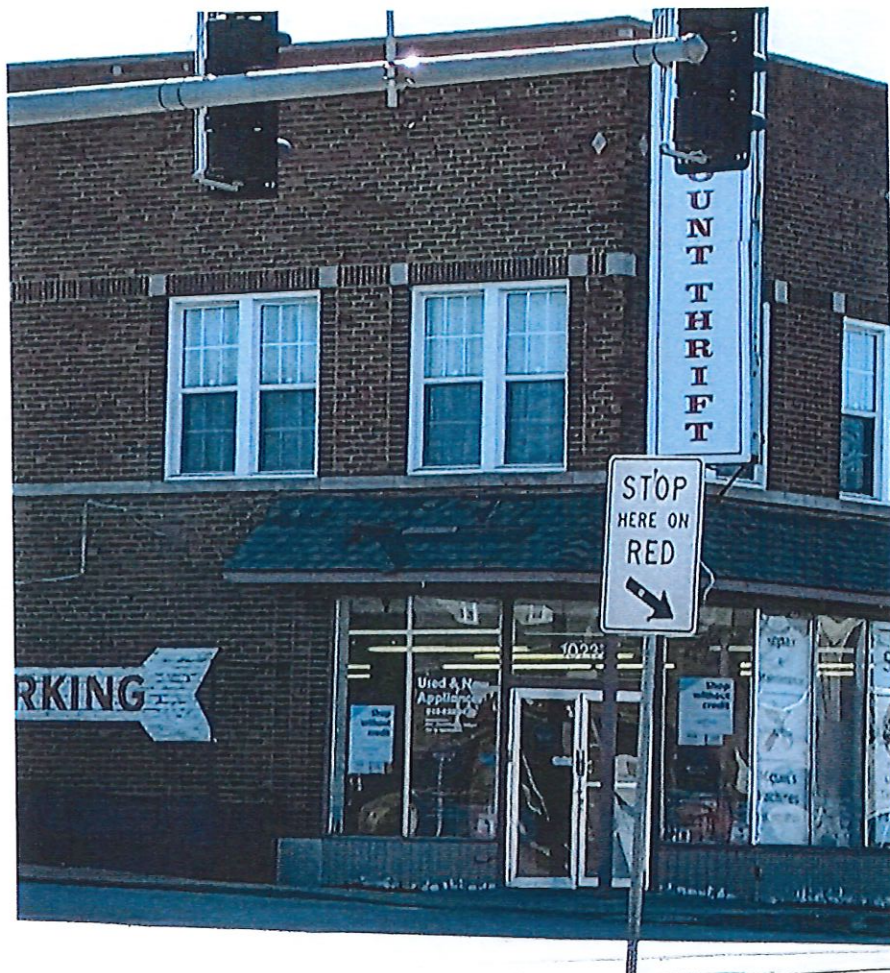
Parcel No. 27-120-08-01-00-0-00-000 Roofing in need of replacement. Façade in need of repair.
