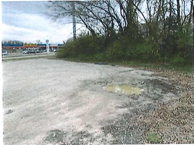
Parcel No. 26-310-04-04-01-0-00-000 Gravel parking lot with pothole
