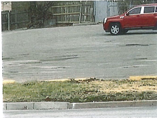
Parcel No. 15-940-10-00-0-00-000 Broken pavement in parking lot
