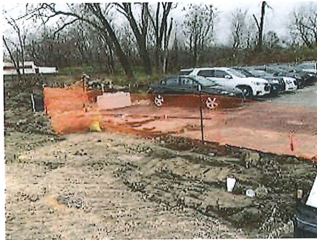
Parcel No. 26-320-05-03-00-0-00-000 Parking lot in disrepair
