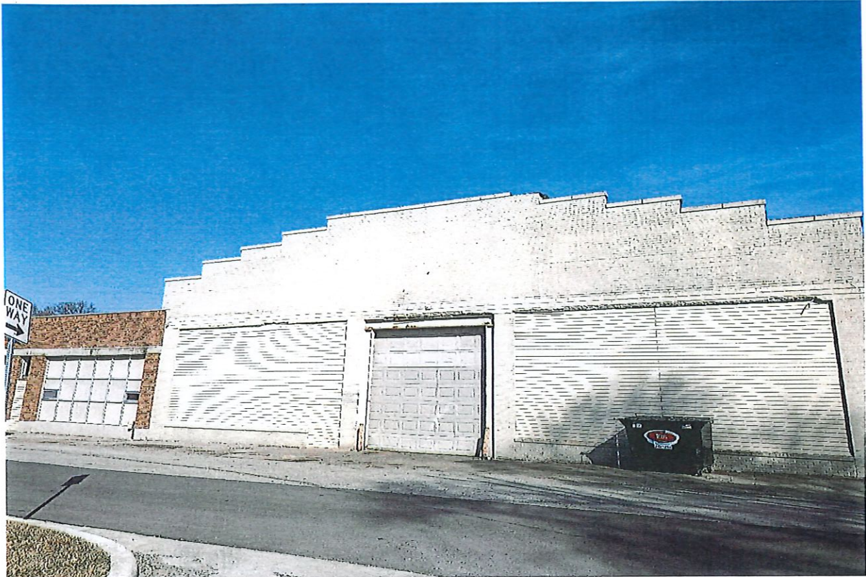
Parcel No. 27-120-06-77-00-0-00-000 Façade in need of improvement. #2
