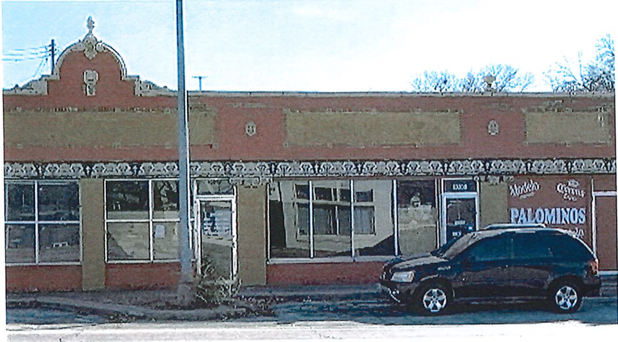
Parcel No. 27-120-08-33-00-0-00-000 Curb deteriorating. Facade in disrepair.
