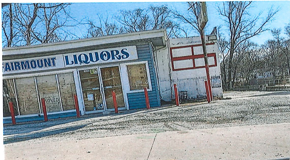
Parcel No. 27-120-01-24-00-0-00-000 Building boarded up and in need of repair.
