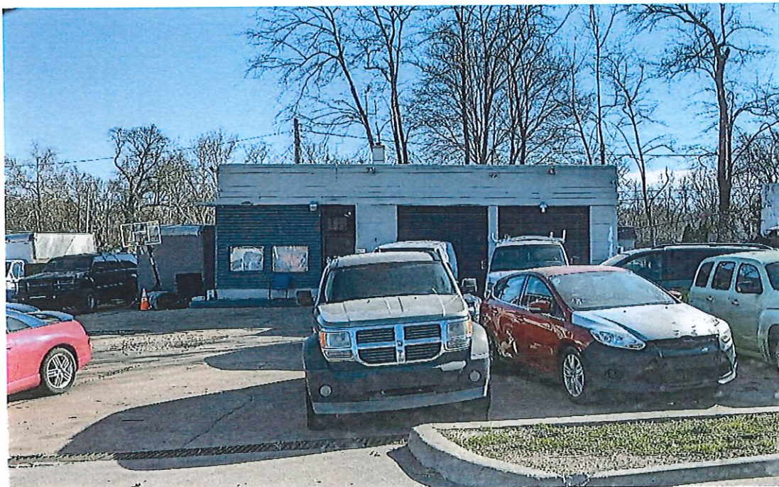
Parcel No. 27-120-02-02-00-0-00-000 Façade in need of repair. Parking lot and curbing deteriorating.
