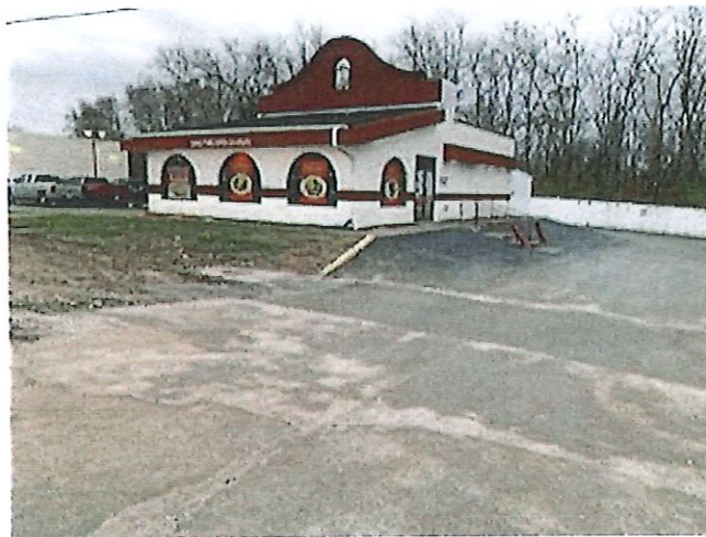
Parcel No. 26-320-05-08-00-0-00-000 Broken pavement
