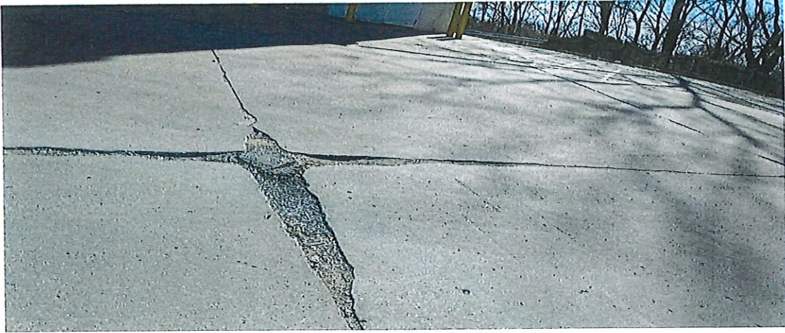
Parcel No. 27-110-04-42-00-0-0-00-000 Poor Condition of parking lot.
