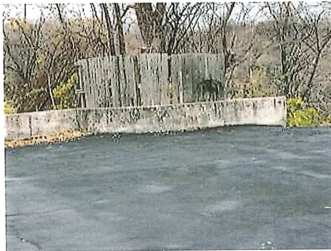
Parcel No. 27-110-02-06-01-0-00-000 Trash enclosure in disrepair
