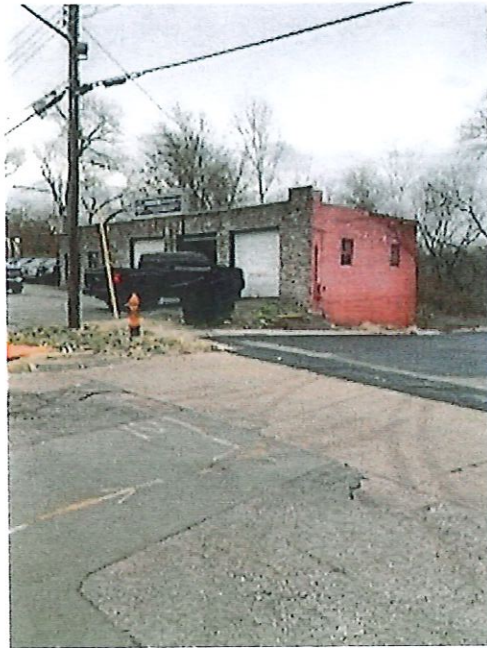
Parcel No. 26-320-05-41-00-0-000 Building in disrepair
