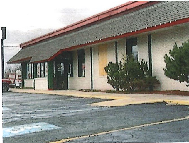
Parcel No. 26-320-05-03-00-0-00-000 Broken window in vacant building
