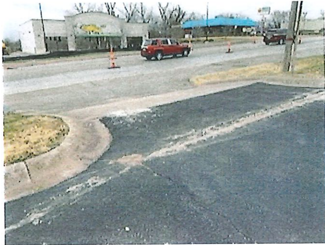
Parcel No. 27-110-02-06-01-0-00-000 Broken driveway
