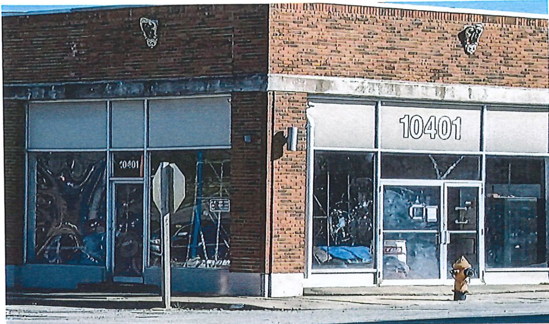
Parcel No. 27-120-06-77-00-0-00-000 Façade in need of improvement. #2
