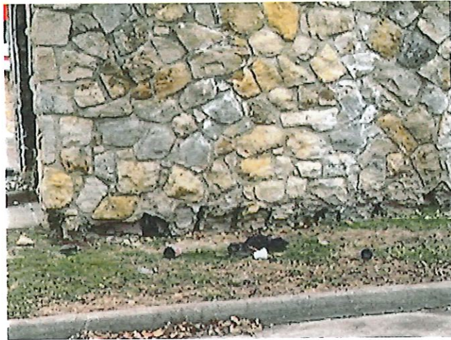
Parcel No. 26-320-05-41-00-0-00-000 Broken wall
