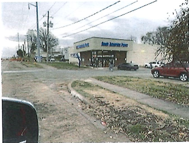
Parcel No. 26-320-05-08-00-0-00-000 Broken Curb
