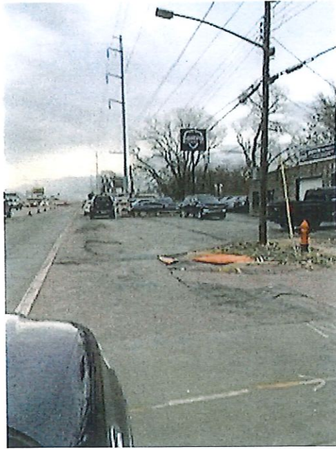
Parcel No. 27-110-21-01-01-0-00-000 27-110-21-01-02-0-00-000 Broken pavement/Cars in right-of-way
