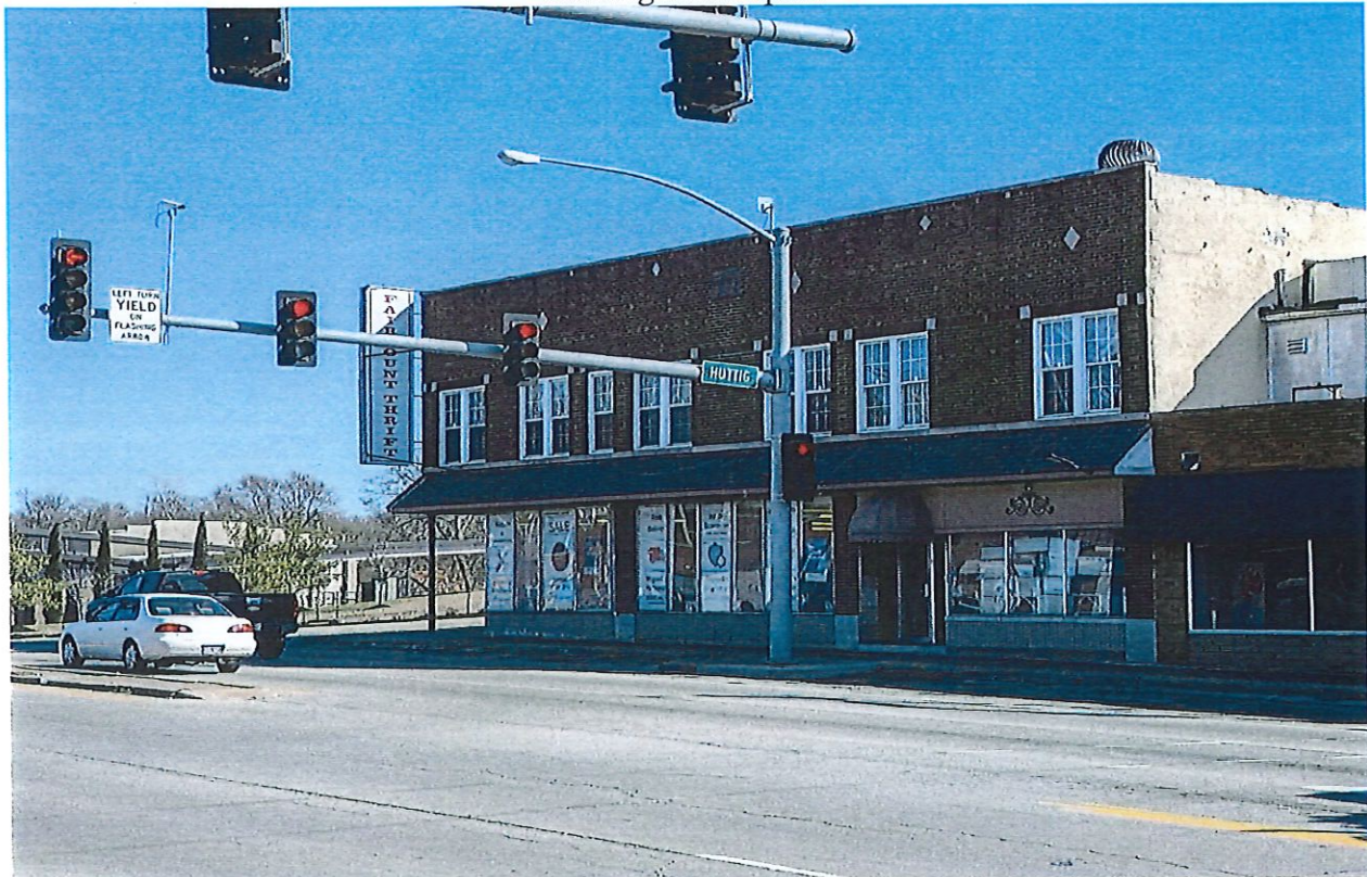
Parcel No. 27-120-08-01-00-0-00-000 Façade in need of repair
