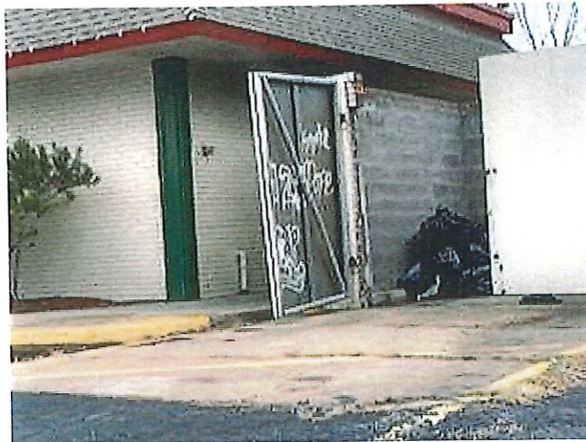
Parcel No. 26-320-05-03-00-0-00-000 Trash enclosure in disrepair
