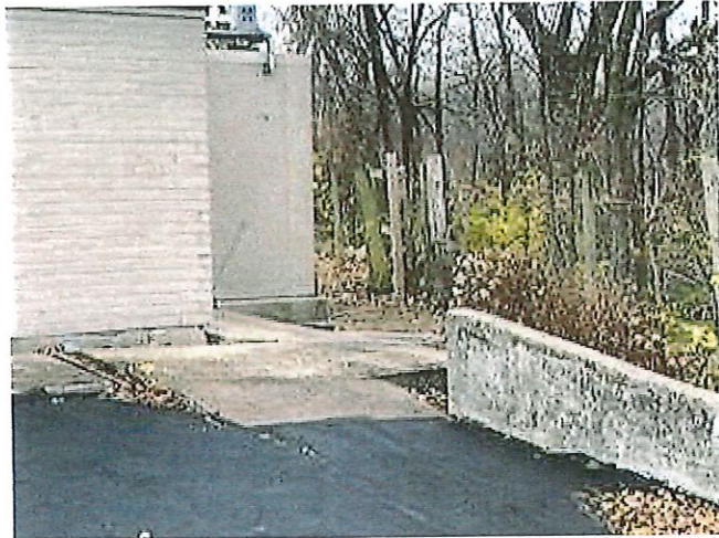
Parcel No. 27-110-02-06-01-0-00-000 Broken fence
