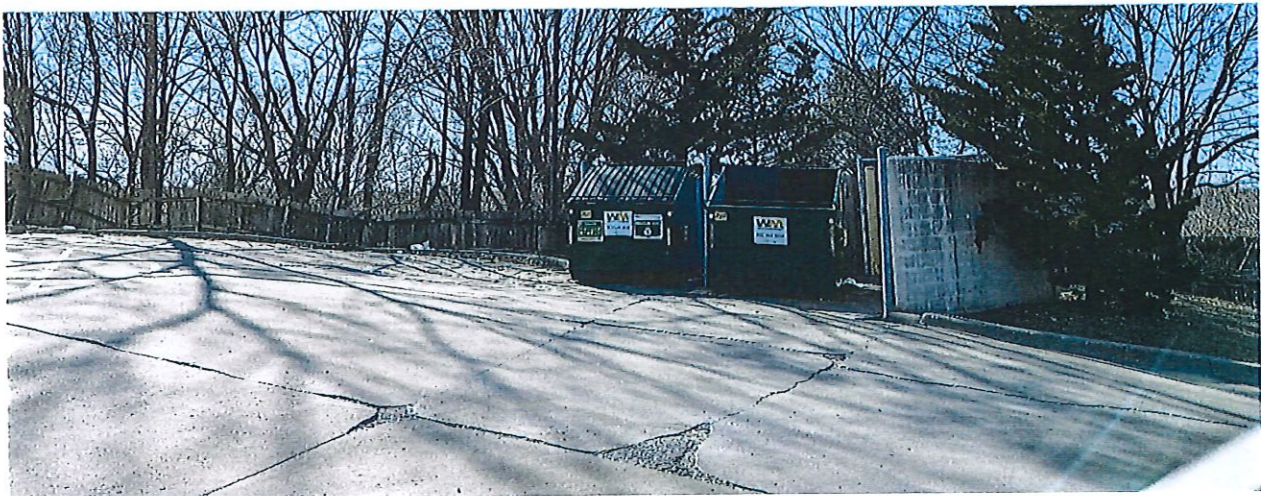
Parcel No. 27-110-04-42-00-0-00-000 Fence broken. Parking lot deterioration
