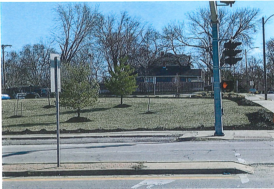
Parcel No. 27-120-07-37-00-0-00-000 Curbing in disrepair.
