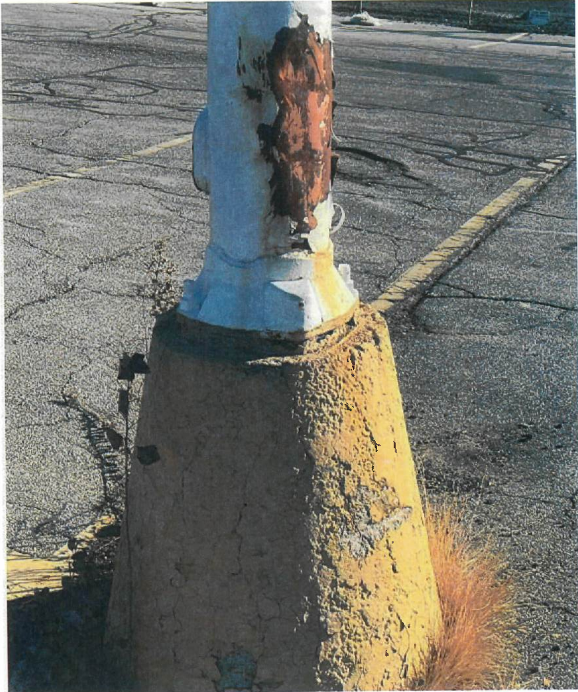
Deteriorated Light Pole
