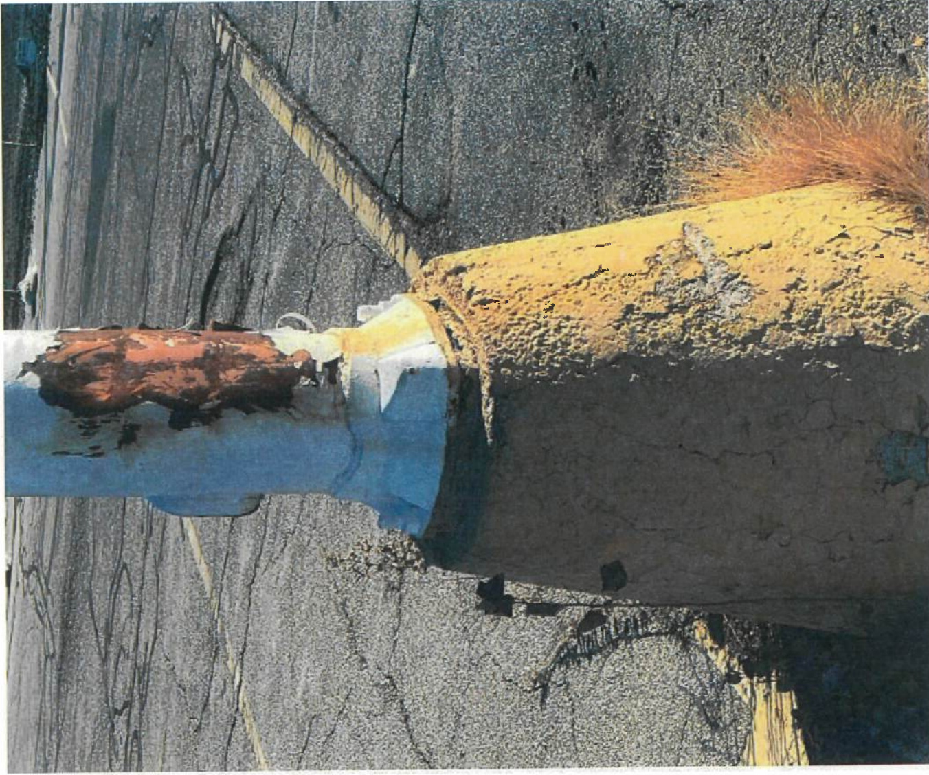
Deteriorated Light Pole
