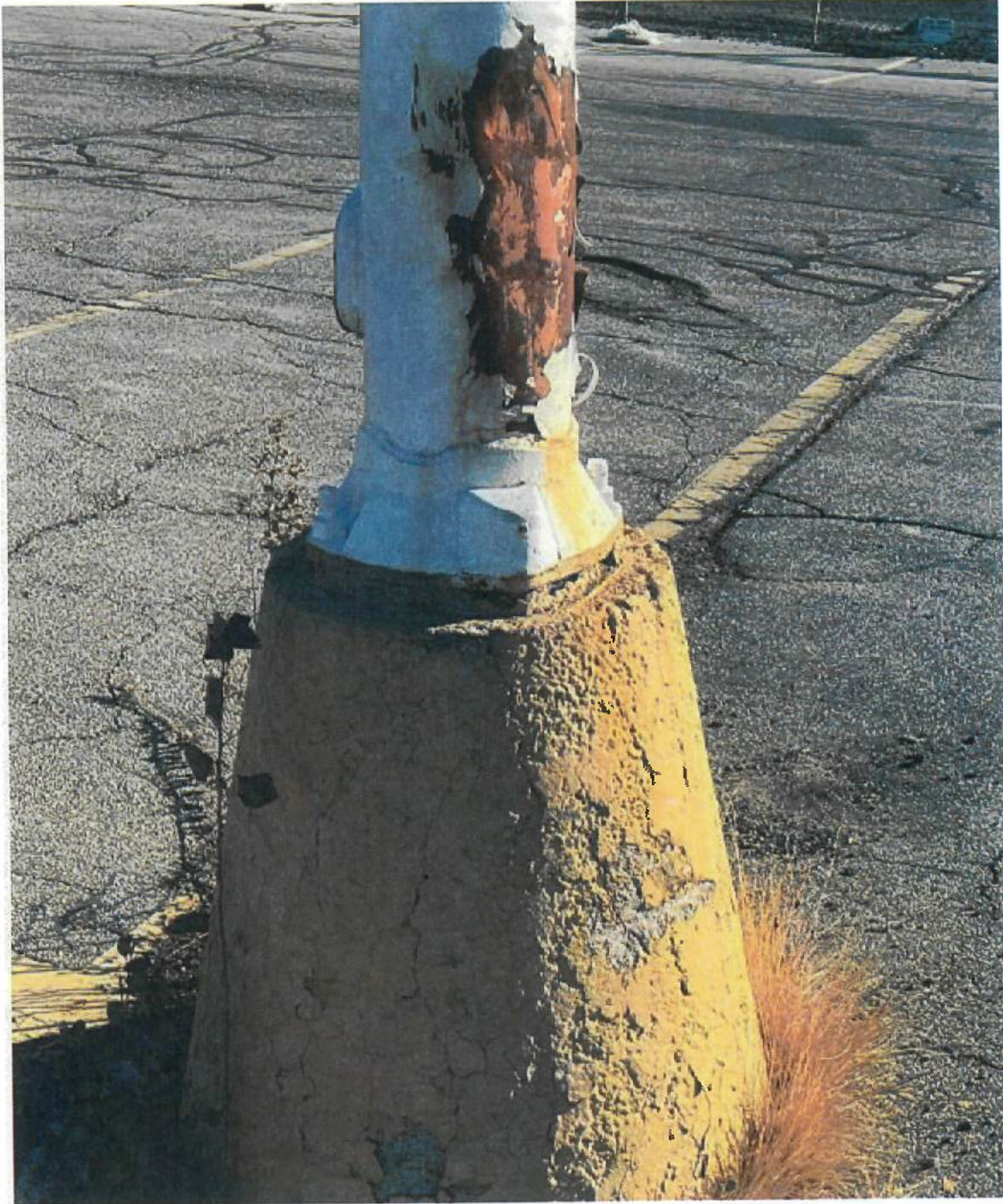
Deteriorated Light Pole
