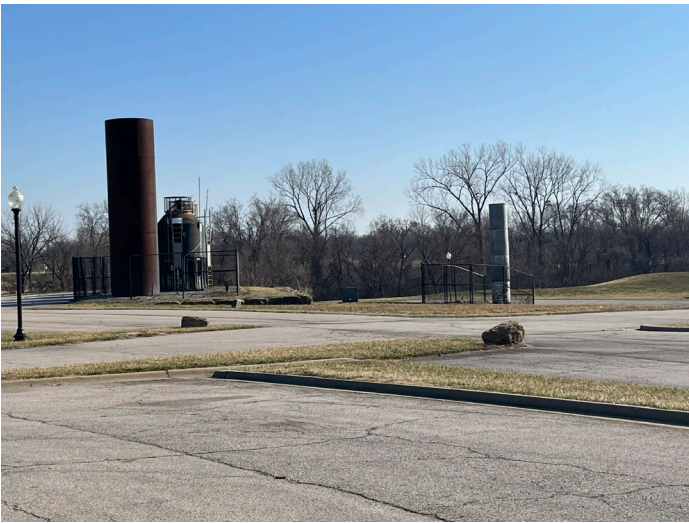
Cave ventilation units fenced off.
