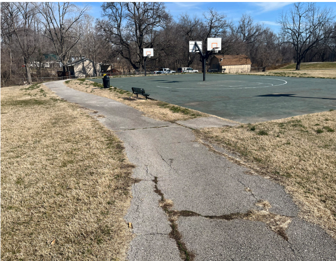
Walkways and basketball courts in aging condition.
