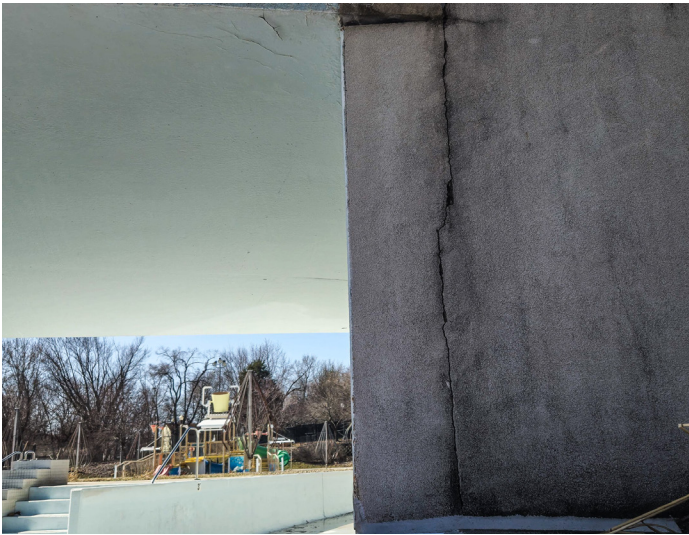
Damaged walking bridge concrete.
