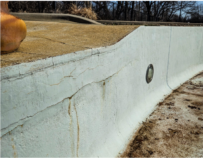
Cracking in pool wall.
