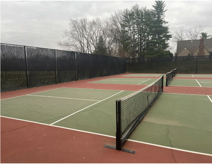
Pickleball court has cracking in the surface.
