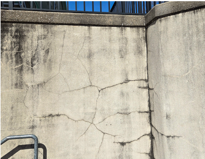
Cracking in pool wall.
