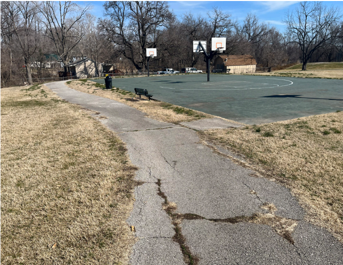
Walkways and basketball courts in aging condition.
