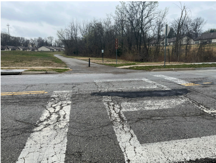
Cross walk with a lack of pedestrian crossing signals.
