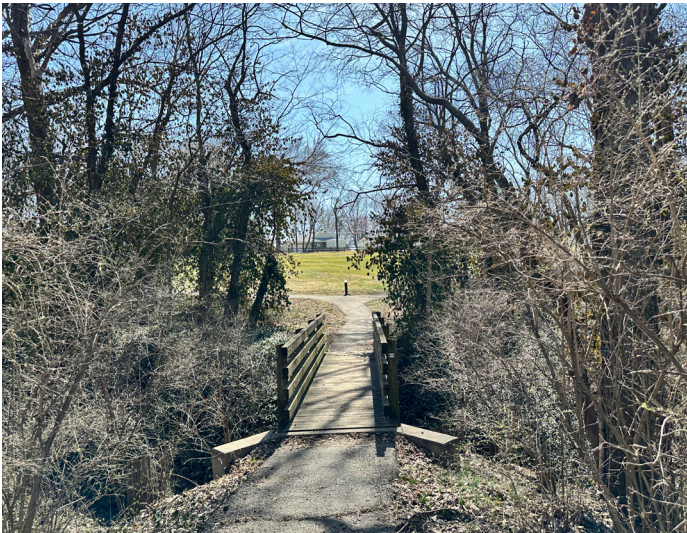
Bridge to park portion of estate in fair condition.
