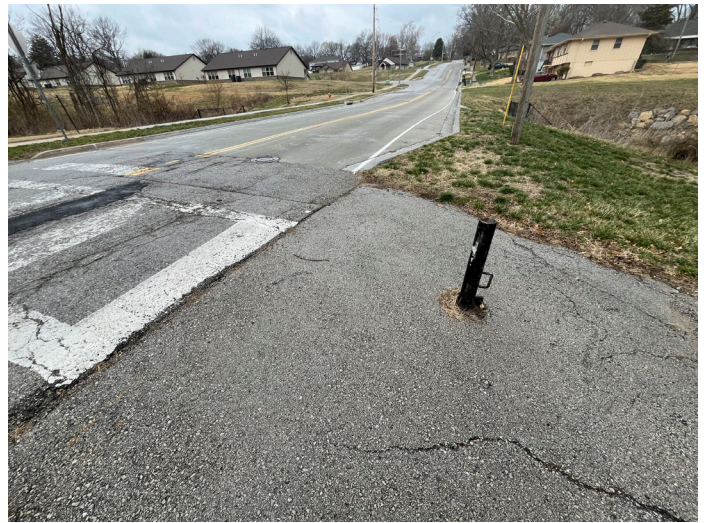
Trail conditions have some cracking and lack some pedestrian amenities.
