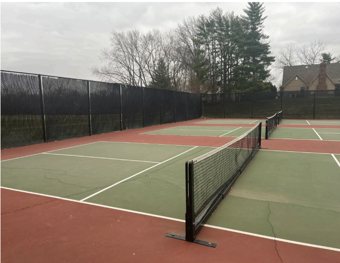
Pickleball court has cracking in the surface.
