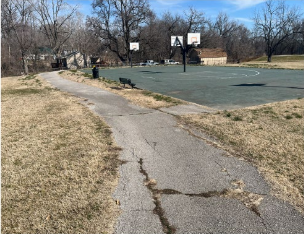
Walkways and basketball courts in aging condition.
