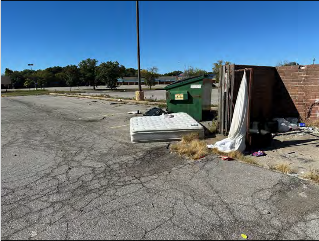
Illegal dumping; deterioration of pavement, trash enclosure; trash/debris
