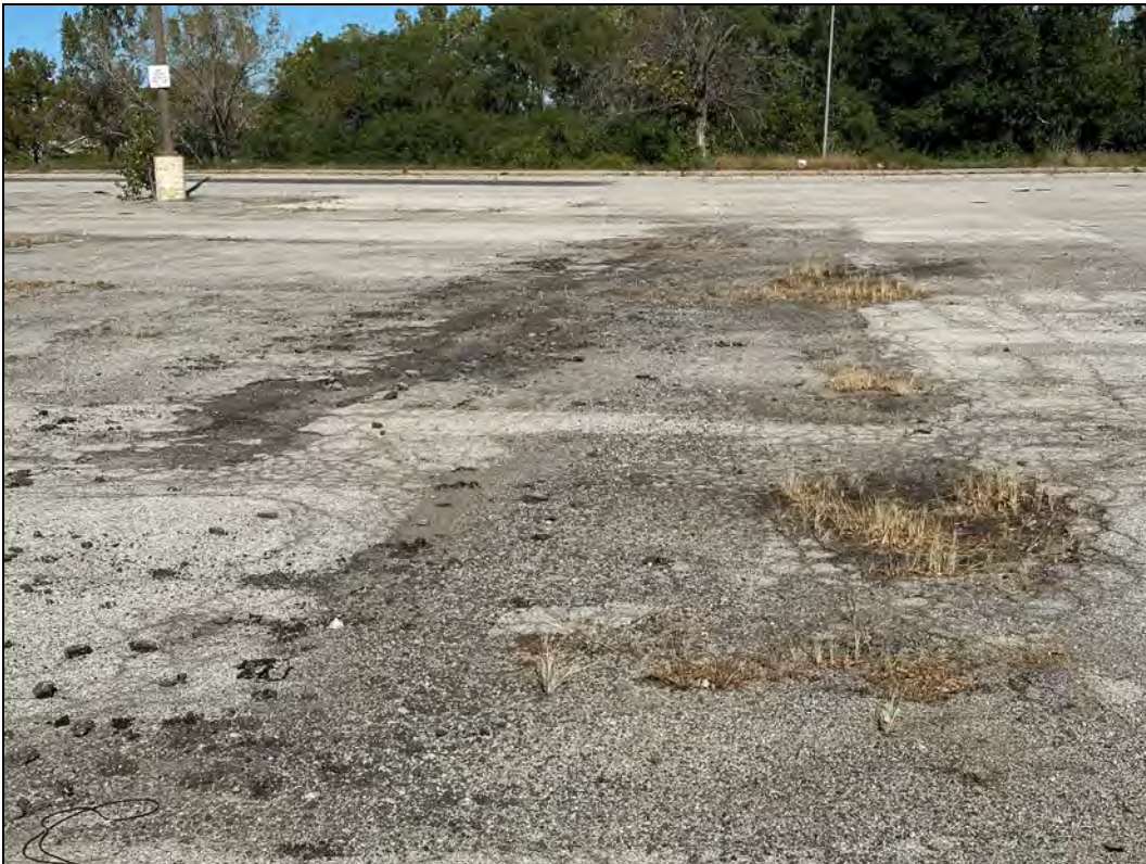
Deterioration of pavement
