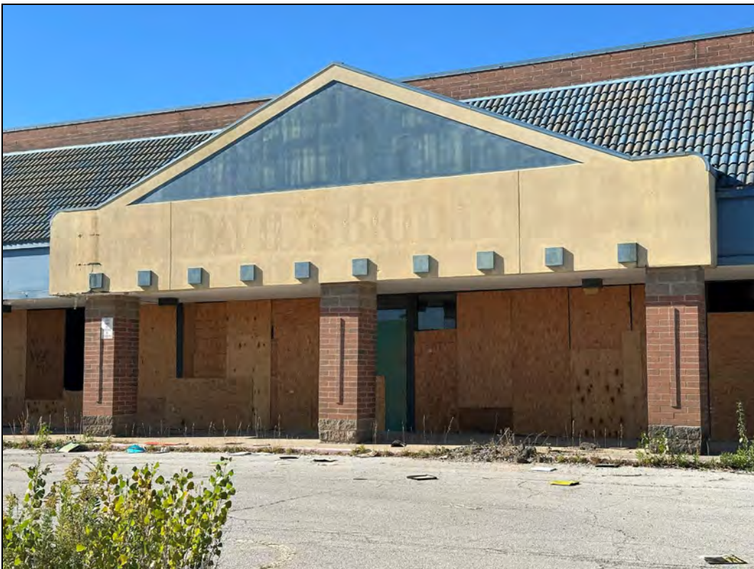
Failure of finishes; boarded windows and doors
