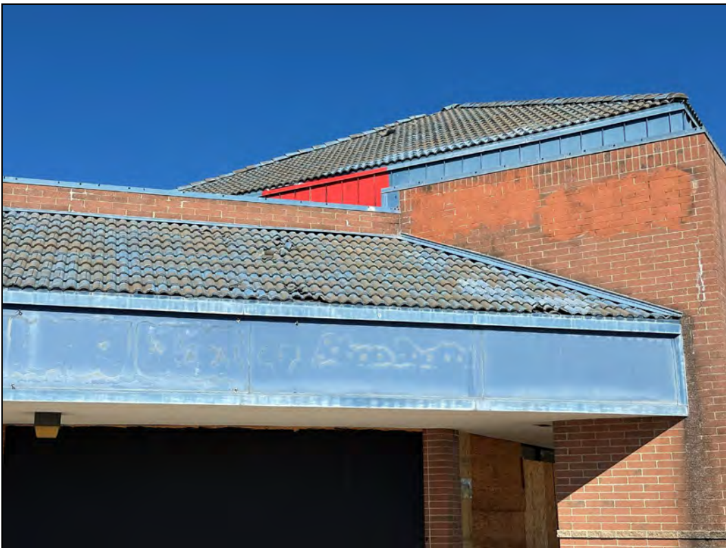
Deterioration of roof; failure of finishes; boarded windows and doors; poor drainage; graffiti
