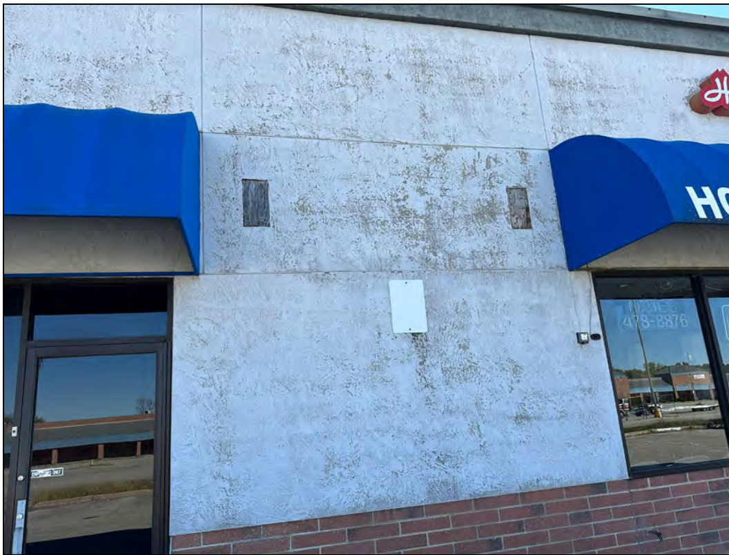
Failure of finishes
