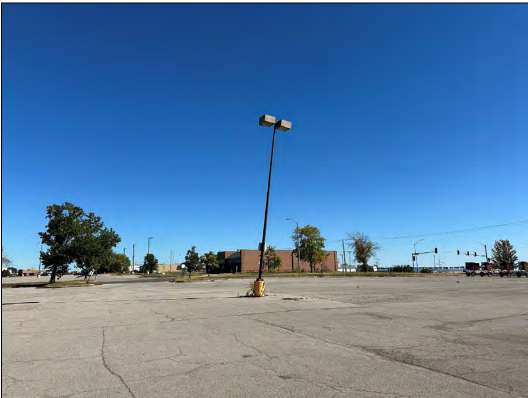
Deterioration of light pole foundation
