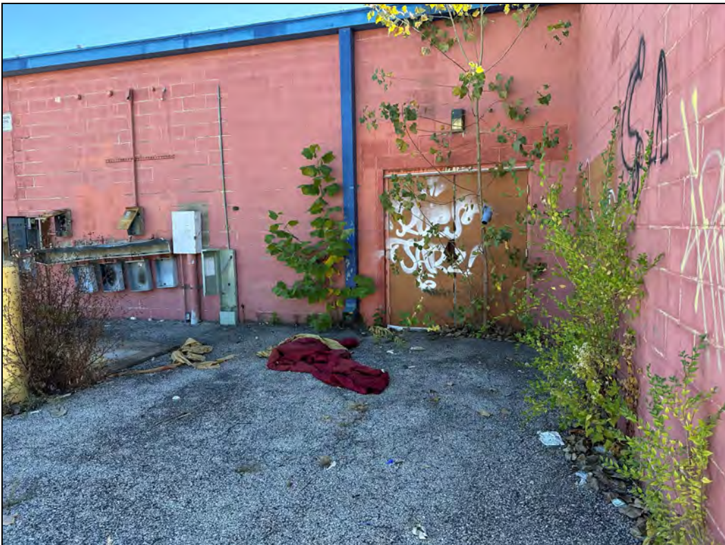
Graffiti; overgrown vegetation; theft of equipment; deterioration of pavement; failure of finishes
