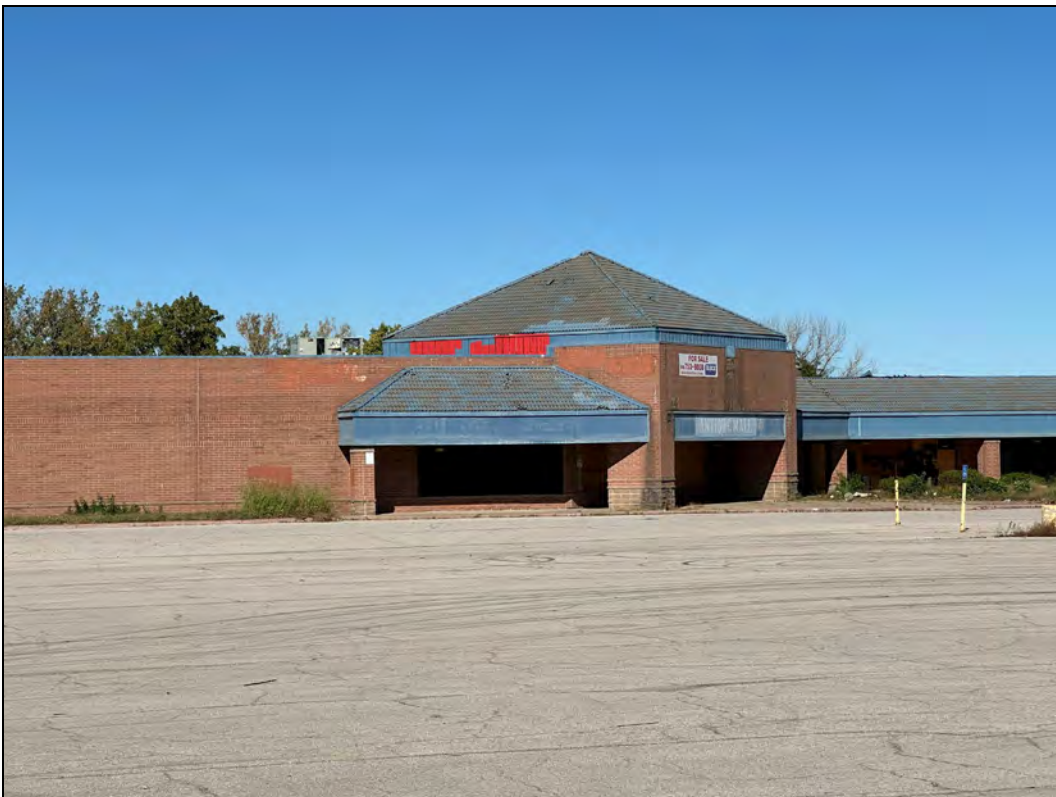
Deterioration of roof; failure of finishes
