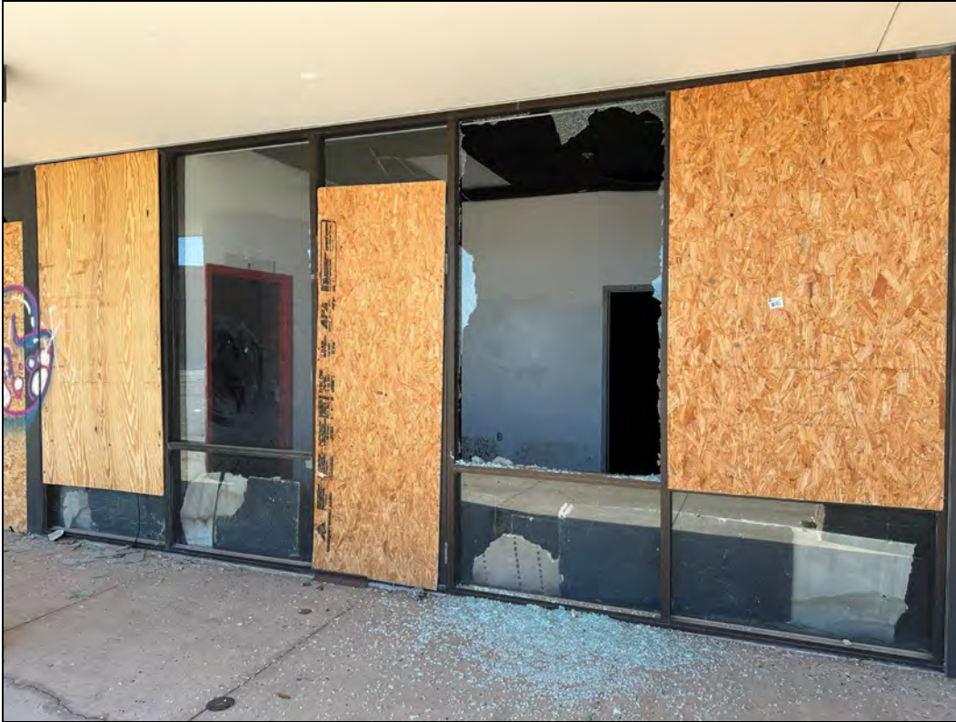
Broken window; glass on sidewalk; boarded windows, doors
