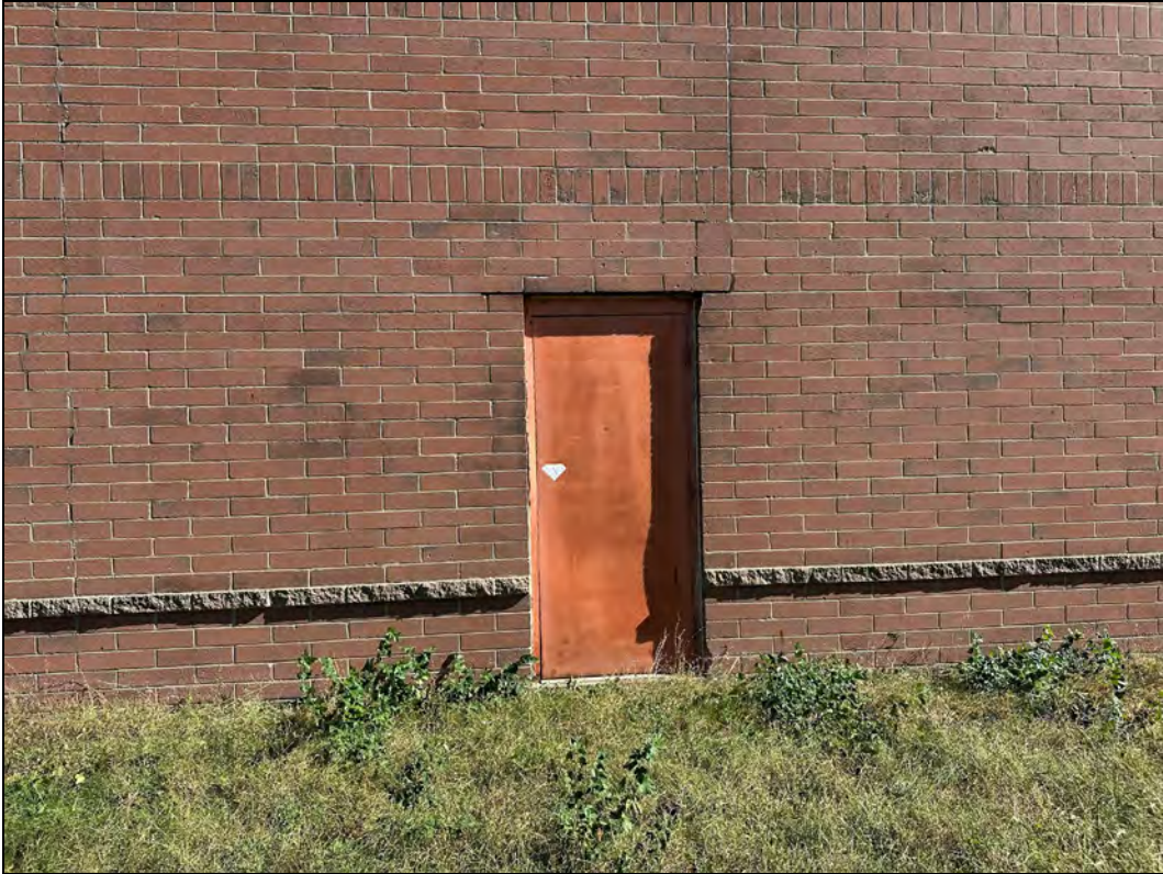
Deterioration of door, lintel; need for mortar repair
