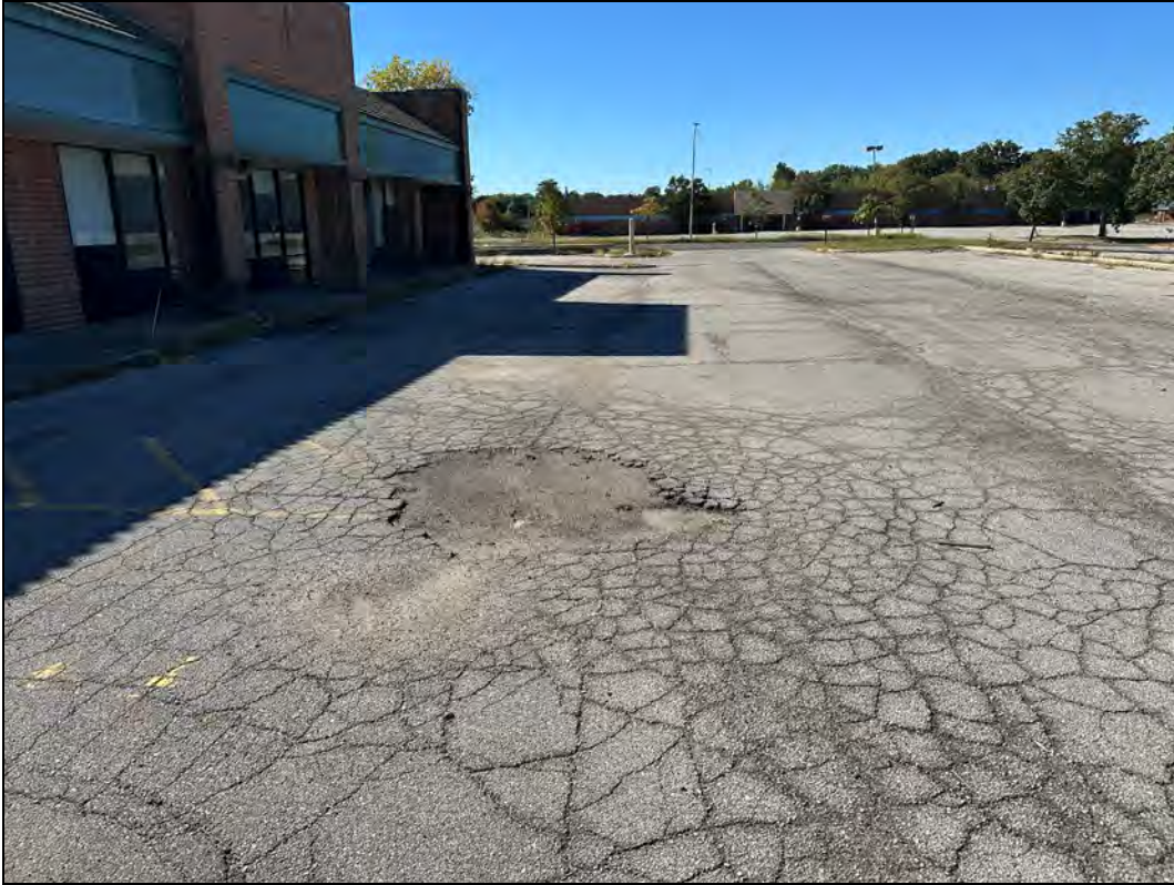
Deterioration of pavement
