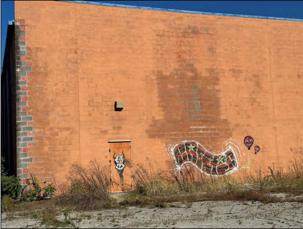
Failure of finishes; deterioration of door; overgrown vegetation; graffiti
