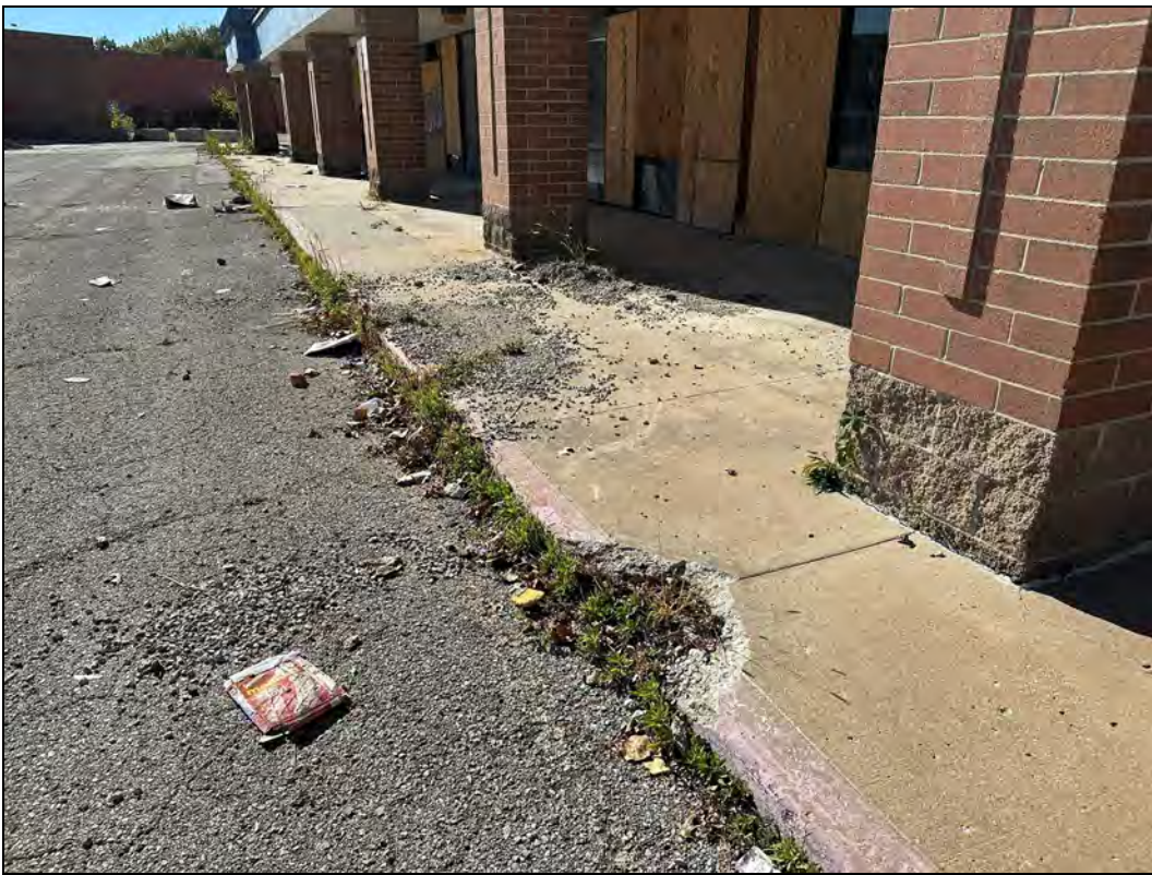
Deterioration of sidewalk, uneven pavement; boarded windows and doors; broken glass on sidewalk
