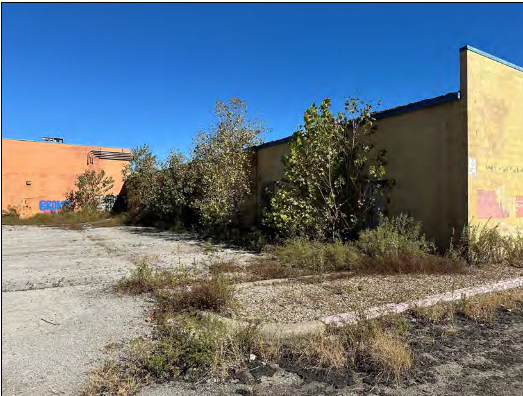
Overgrown vegetation; graffiti; deterioration of pavement; failure of finishes
