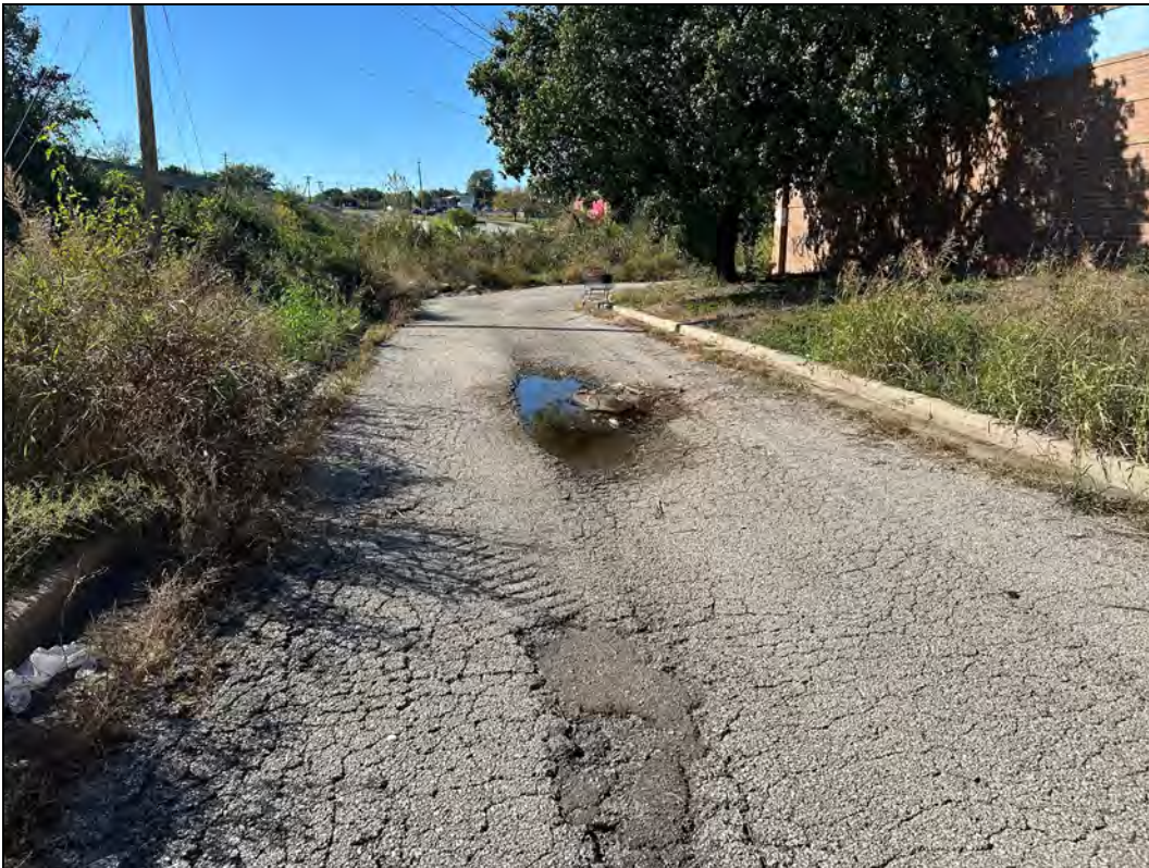
Deterioration of pavement; overgrown vegetation
