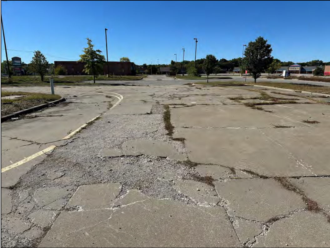
Deterioration of pavement
