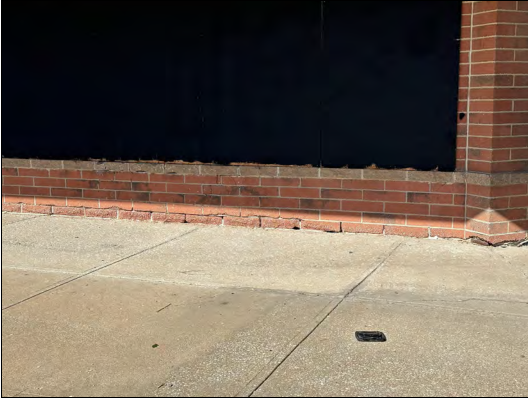
Deterioration of brick veneer; boarded windows
