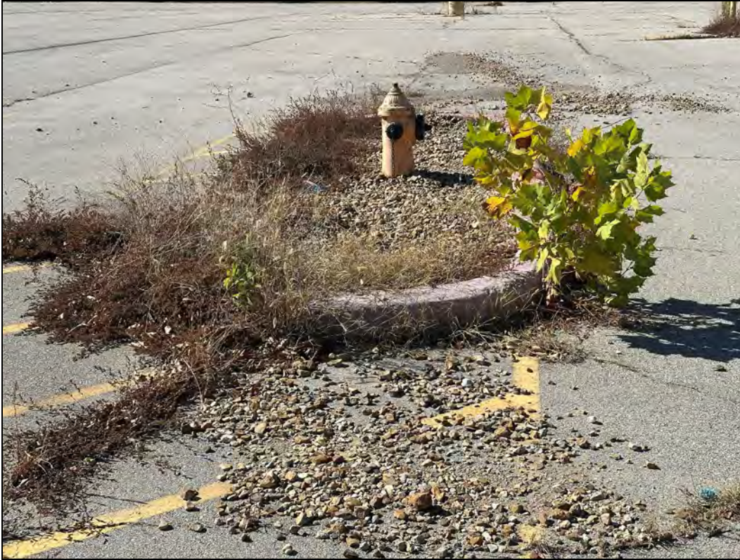
Overgrown vegetation, debris, deterioration of parking lot
