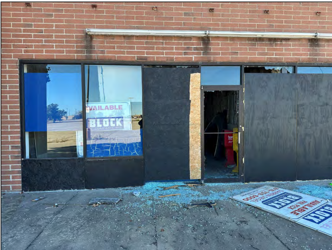
Vandalism (broken glass door); broken glass on sidewalk
