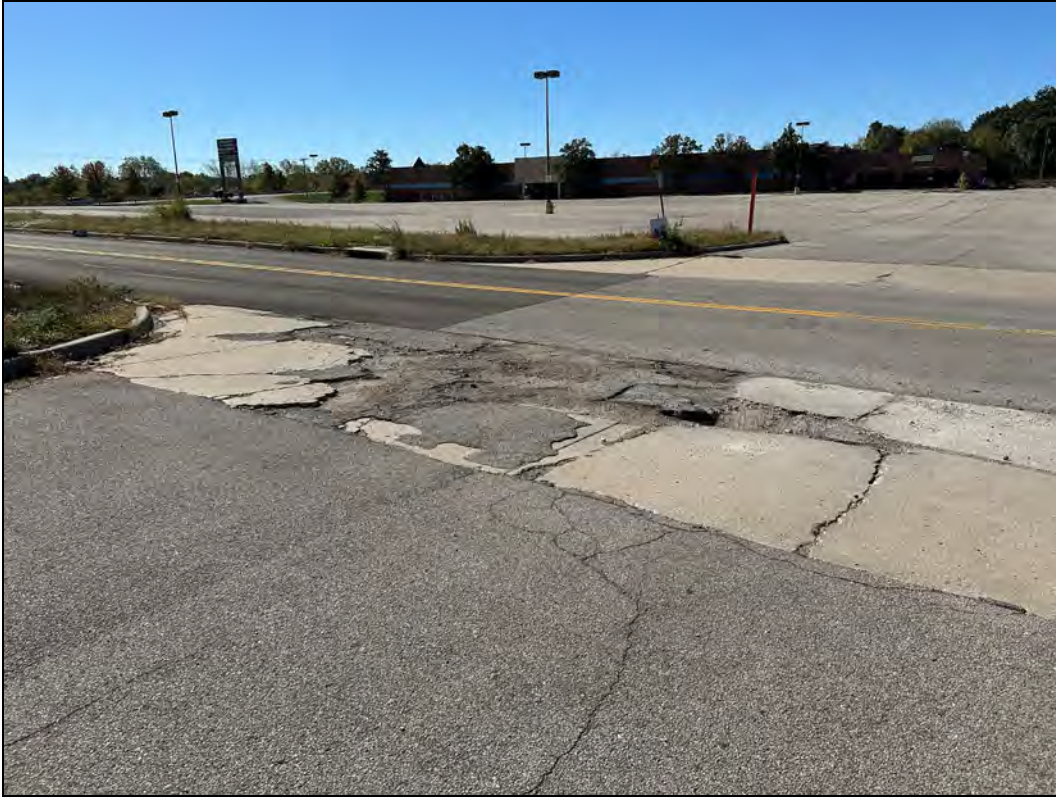
Deterioration of pavement
