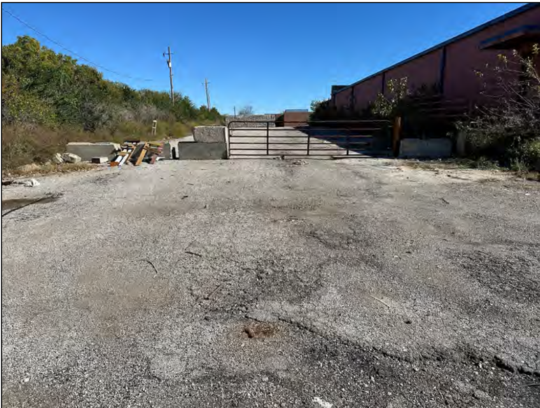
Deterioration of pavement; trash/debris; overgrown vegetation
