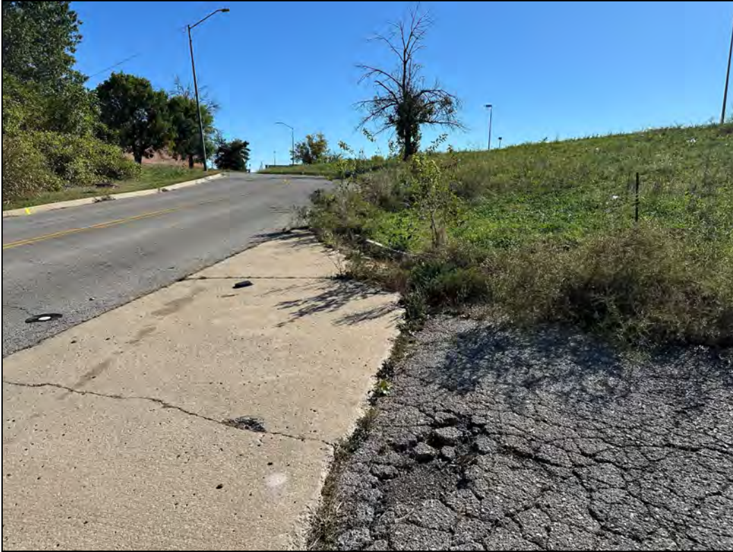
Neglected landscaping; deterioration of pavement
