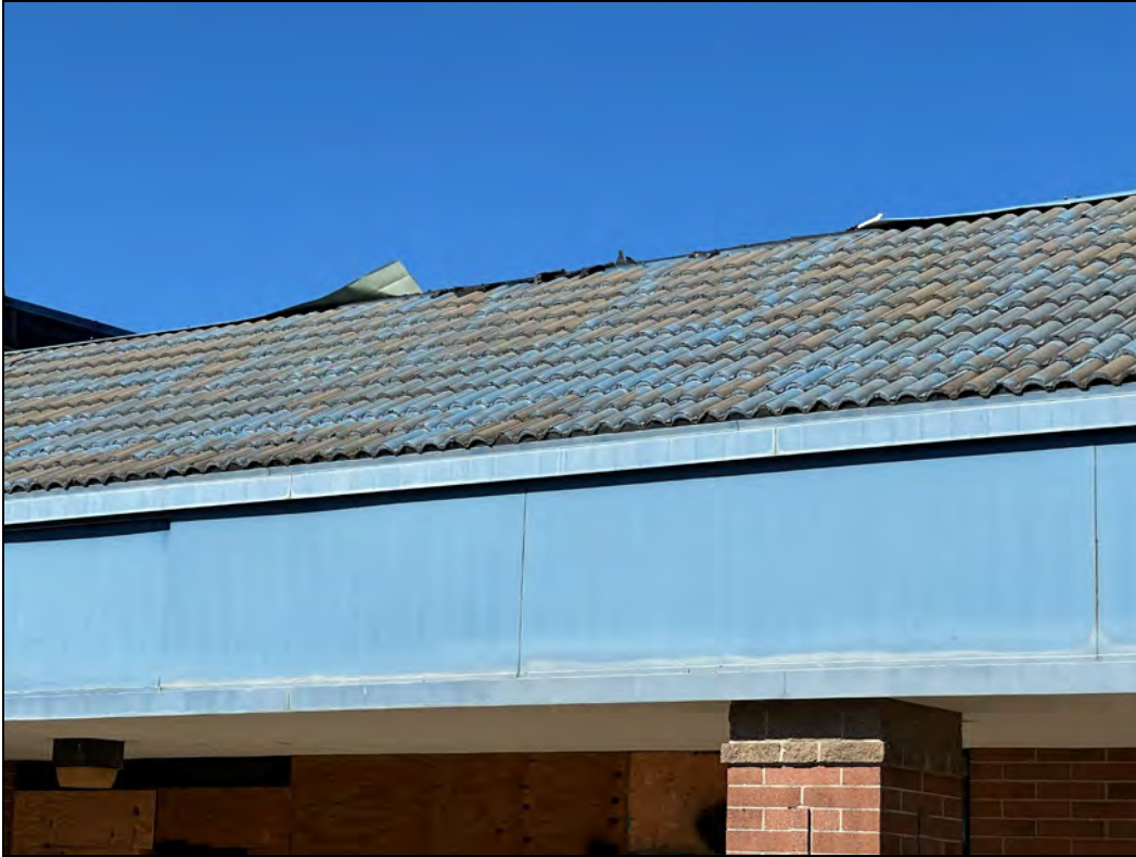
Deterioration of roof; failure of finishes
