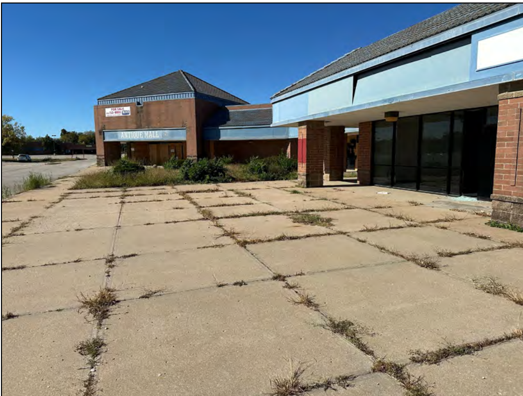
Uneven pavement caused by growth of vegetation; broken glass on pavement
