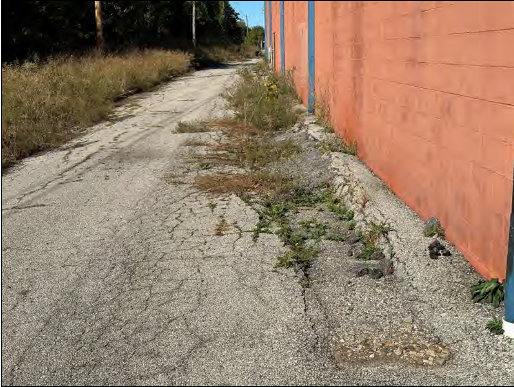
Deterioration of pavement; failure of finishes; overgrown vegetation
