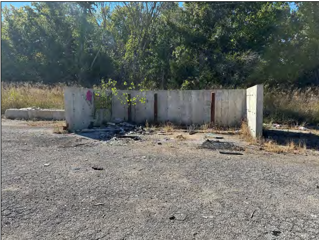
Deterioration of pavement; trash/debris; overgrown vegetation
