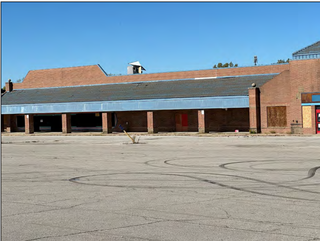
Deterioration of roof-top equipment; failure of finishes
