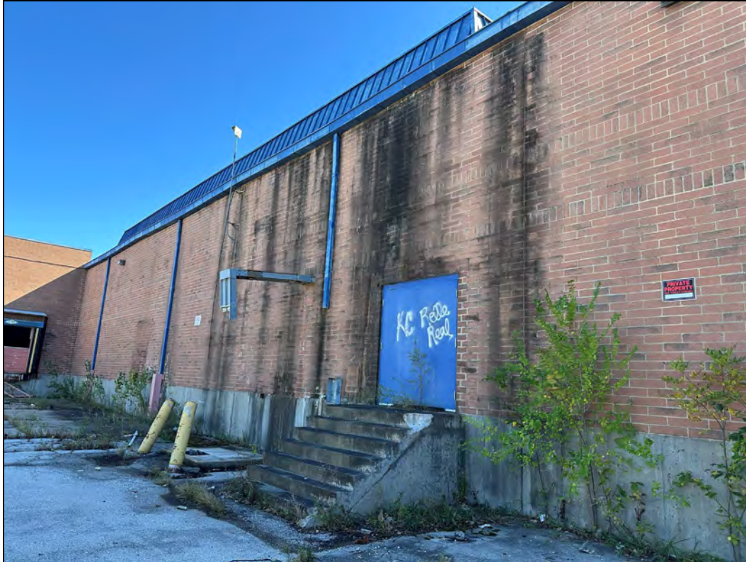
Deterioration of gutter, steps; lack of railing; graffiti; overgrown vegetation; damaged bollards
