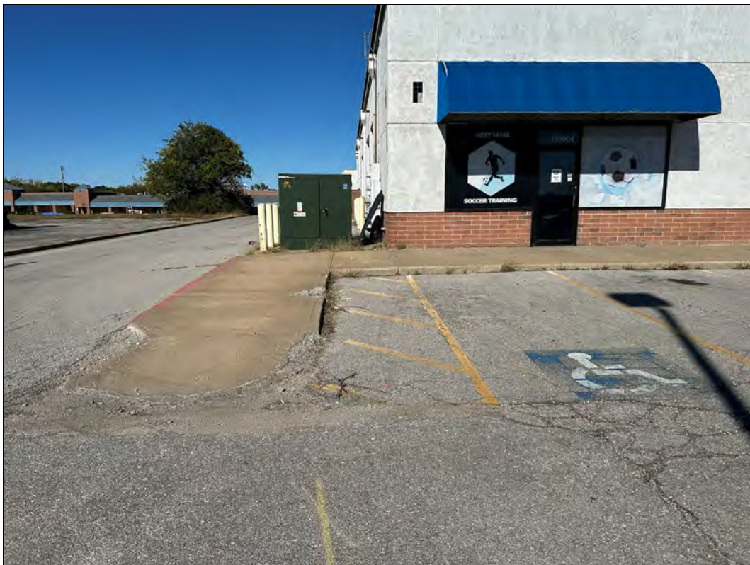
Deterioration of sidewalk; ADA signage, aisle non-compliant; faded pavement markings
