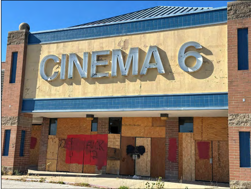
Failure of finishes
