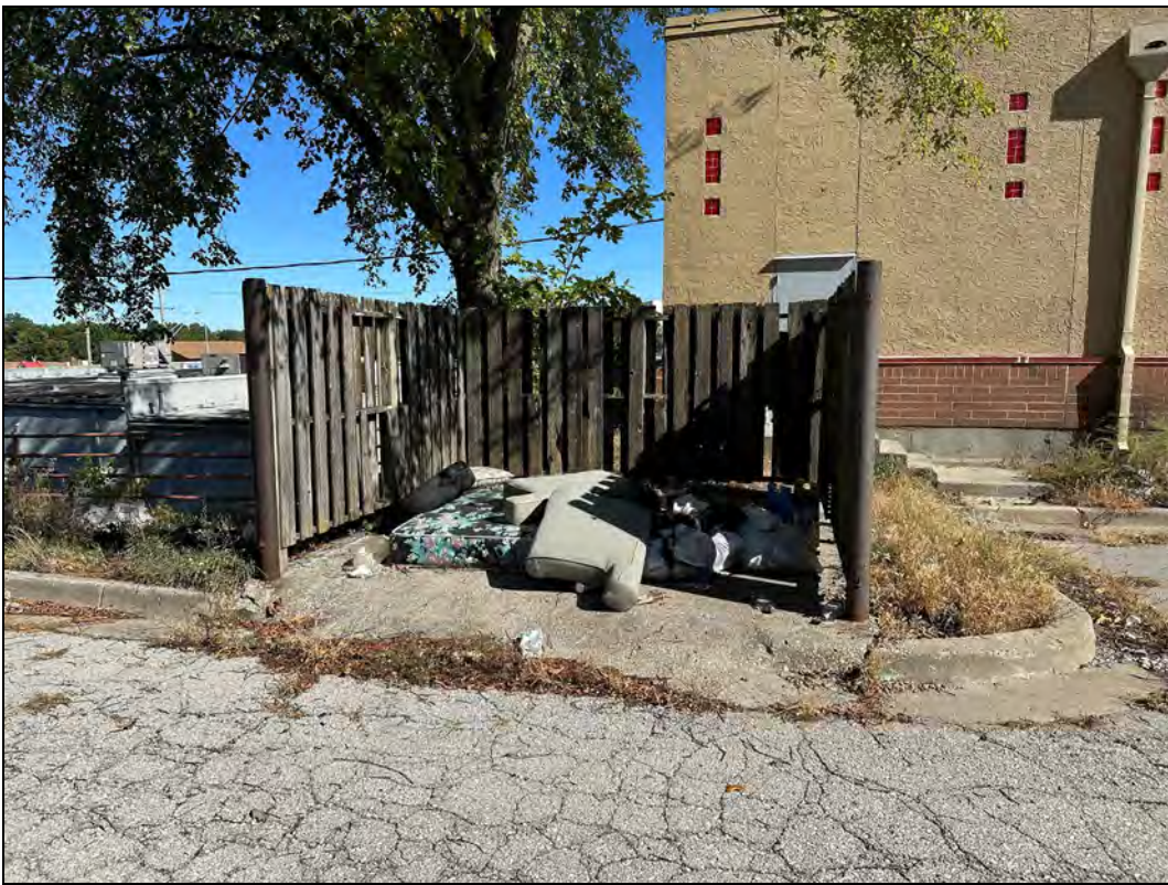
Illegal dumping; deterioration of trash enclosure, pavement
