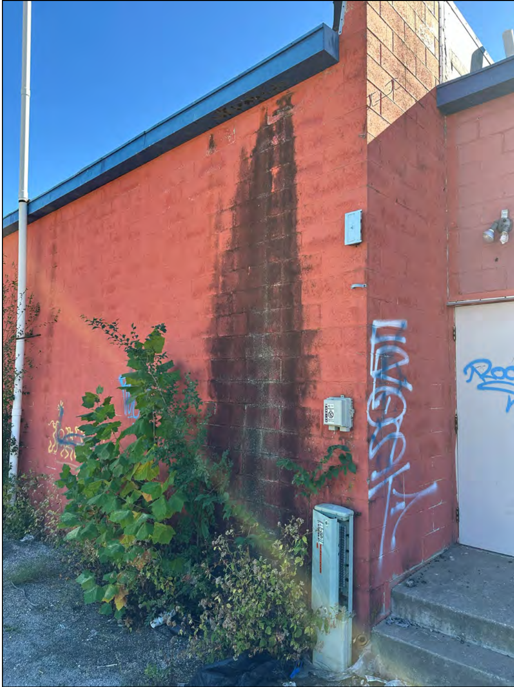
Deterioration of gutter; overgrown vegetation; graffiti; failure of finishes
