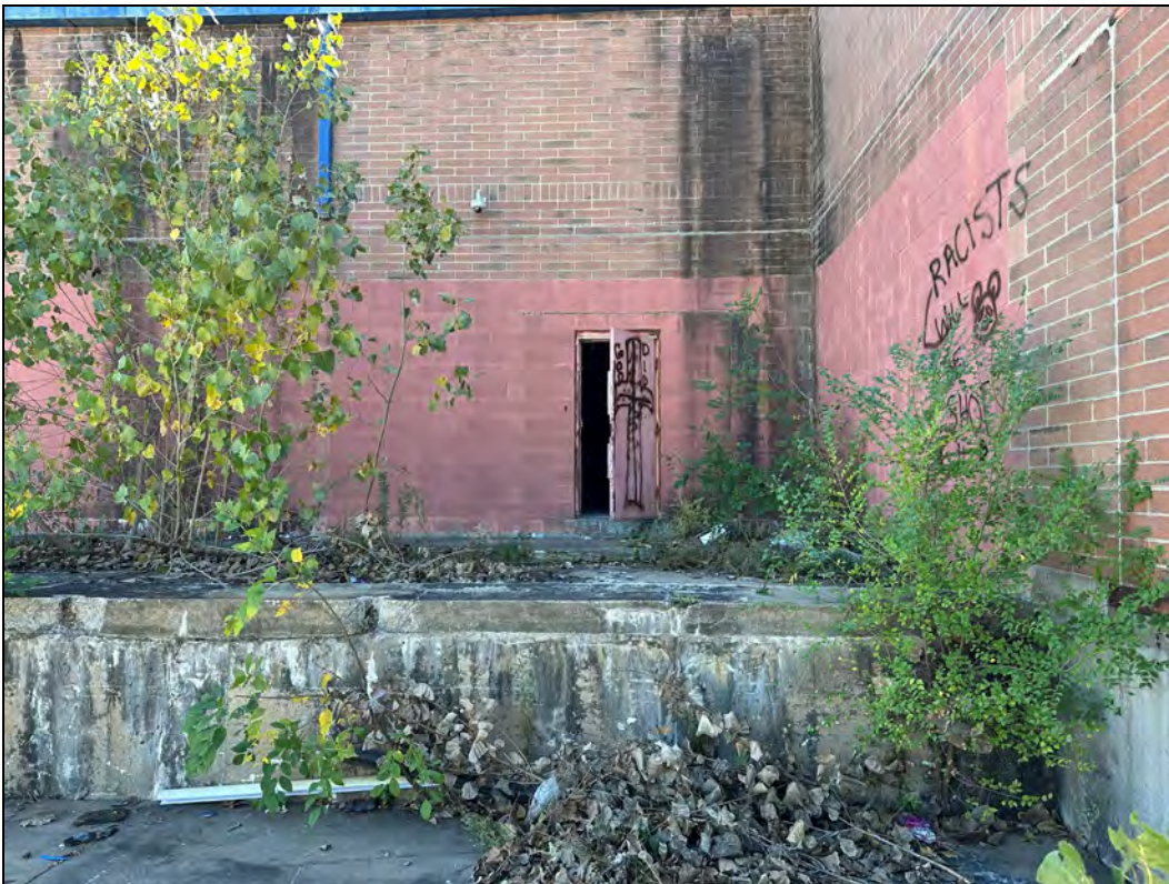
Unsecured access to dangerous building; graffiti; overgrown vegetation; missing downspouts
