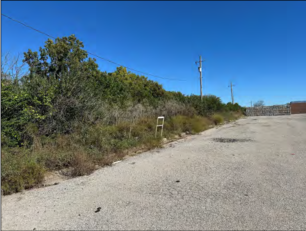
Deterioration of pavement; overgrown vegetation
