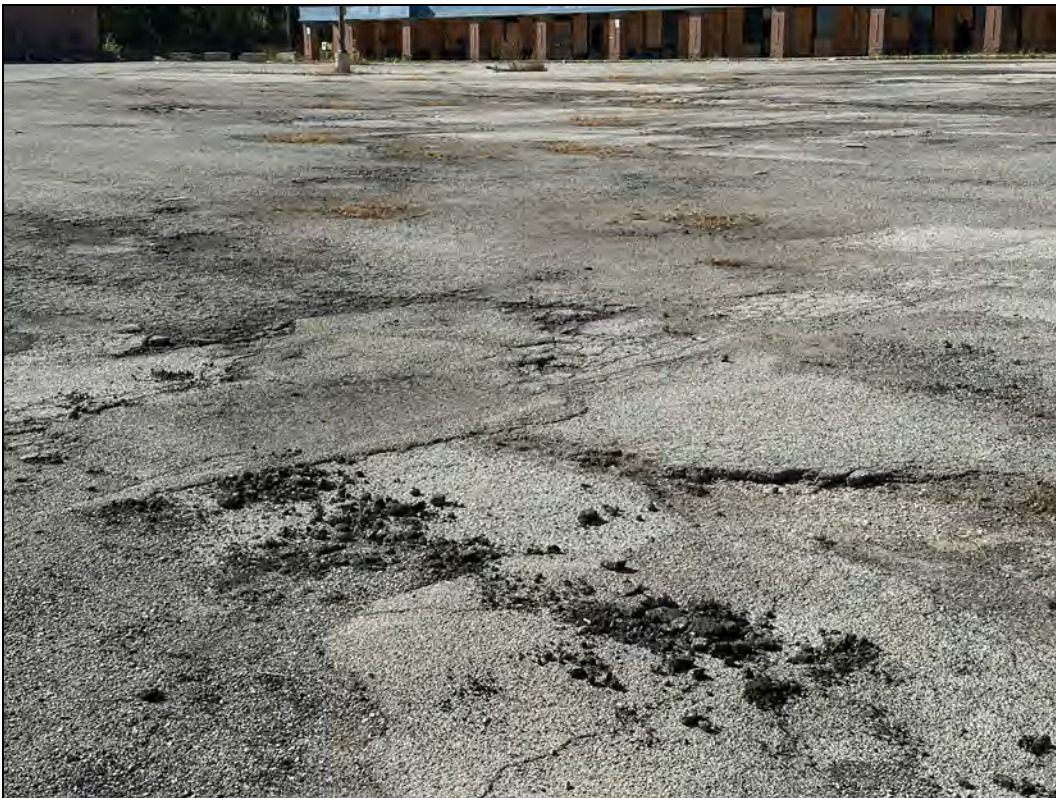
Deterioration of pavement
