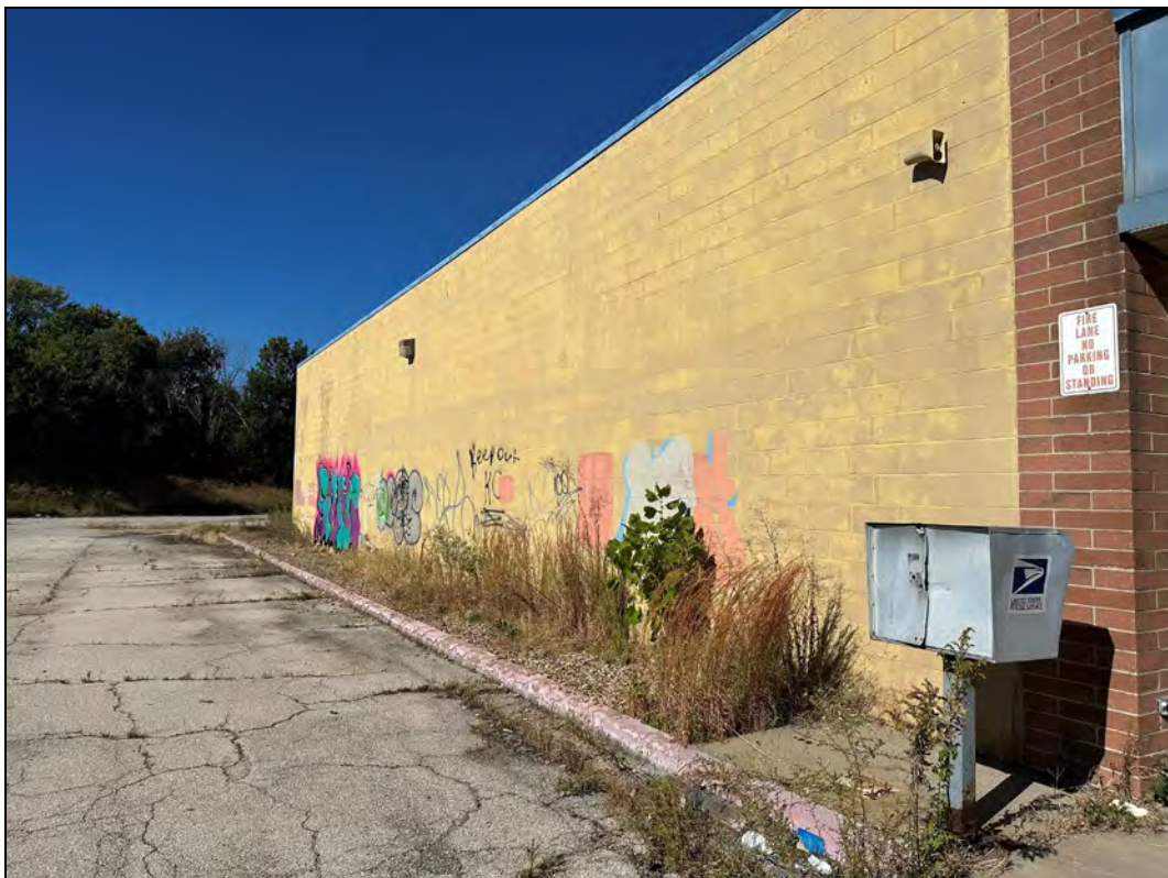
Failure of finishes; graffiti; overgrown vegetation; deterioration of pavement
