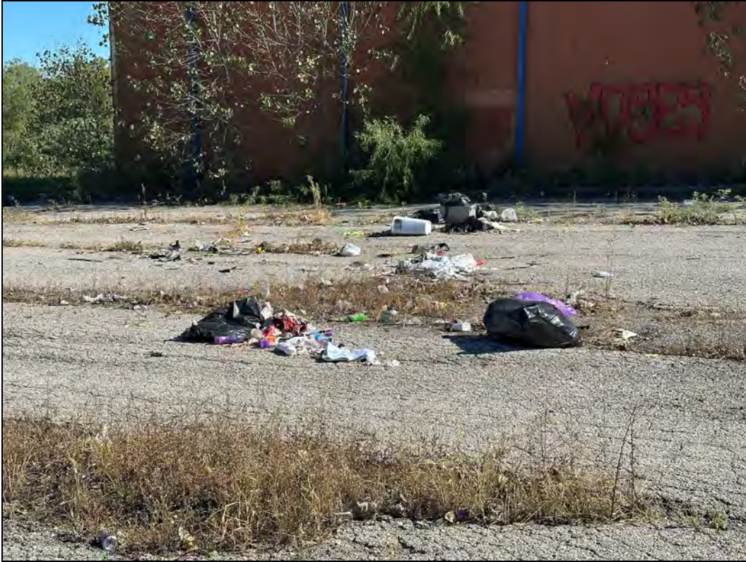
Deterioration of pavement; overgrown vegetation; trash/debris
