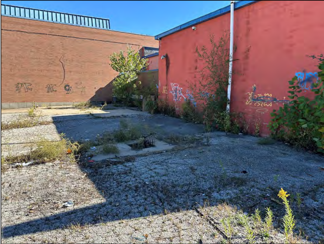
Graffiti; overgrown vegetation; deterioration of pavement
