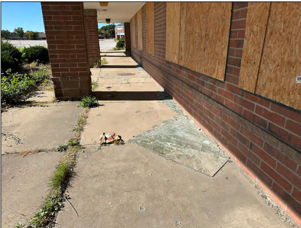
Unsafe/uneven sidewalk caused by vegetation growth, debris, broken glass
