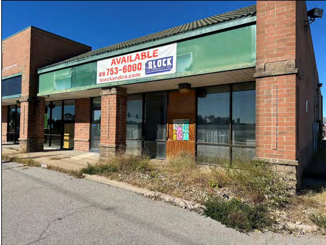
Failure of finishes; overgrown vegetation; boarded door
