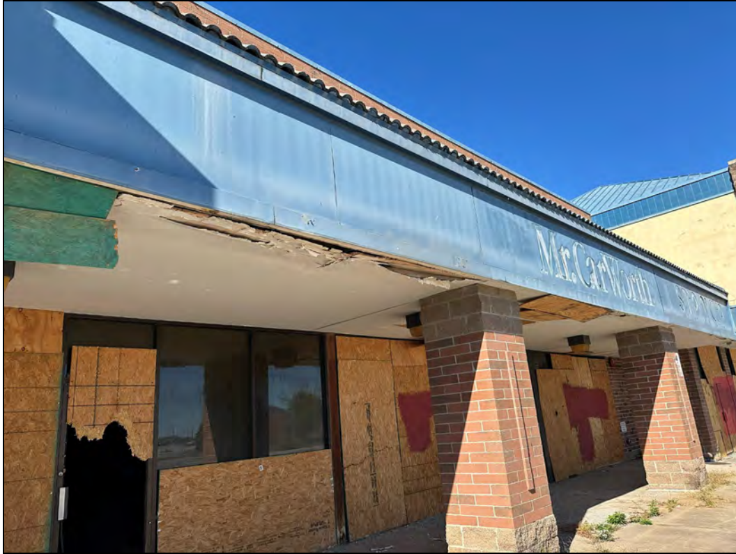
Open access to dangerous building; boarded windows and doors; failure of finishes; deterioration of soffit
