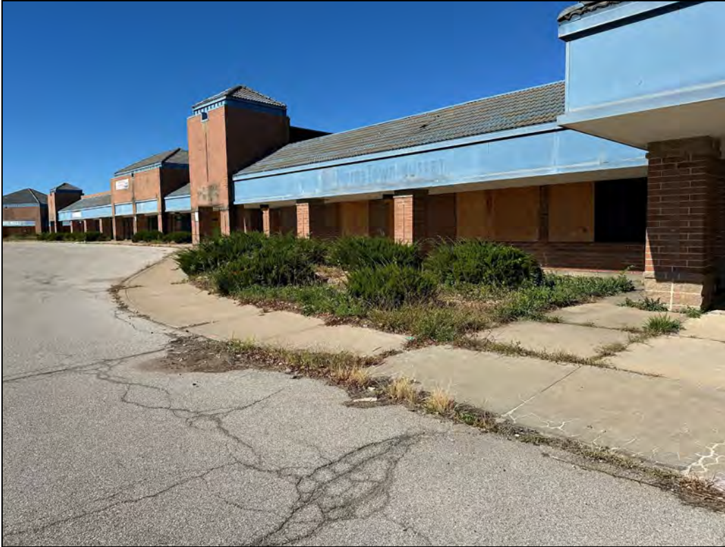
Deterioration of sidewalk; uneven pavement due to growth of vegetation; overgrown vegetation
