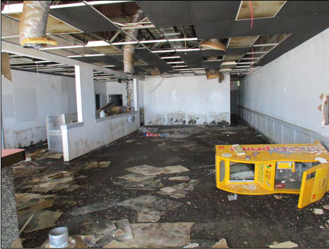
Mold; trash/debris; disconnected/nonfunctioning building systems
