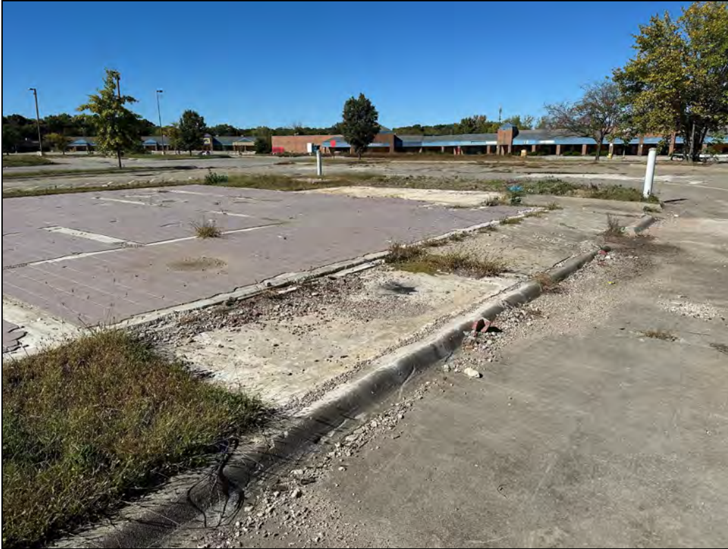
Deterioration of sidewalk, pavement
